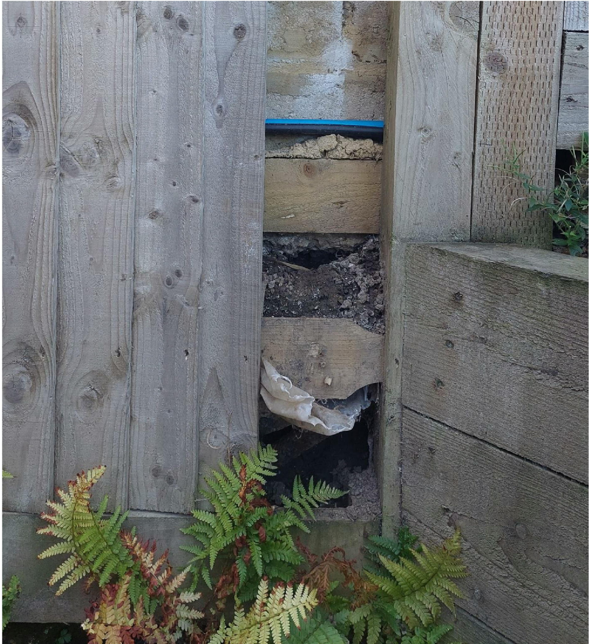
Figure 3: Close up of soil and plastic fill below the blue pipe. The horizontal timber board that has been fixed to the back of the fence is visible just below the blue pipe.
