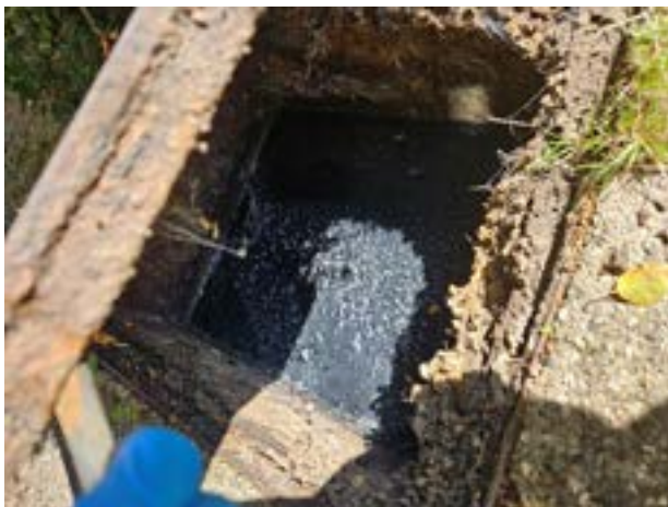
Blocked drains on arrival
