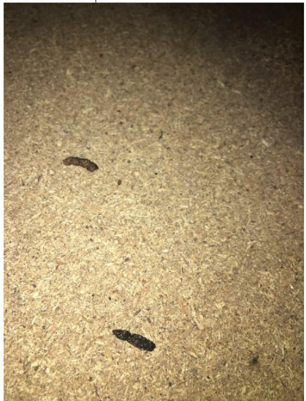
Bat droppings on top of water tank
