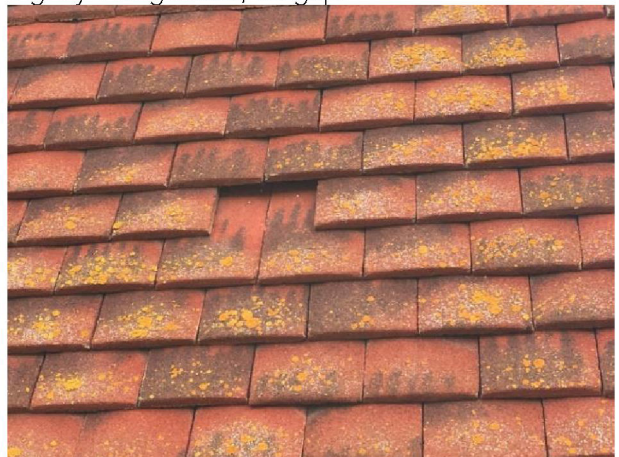
Occasional missing hanging tiles
