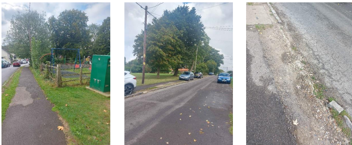
Figure 3. 3 photos showing the playground at the south end of Bowers Place, the road and condition of the verge and kerb. Taken by Luke Davenport on the 3rd of September 2024.
