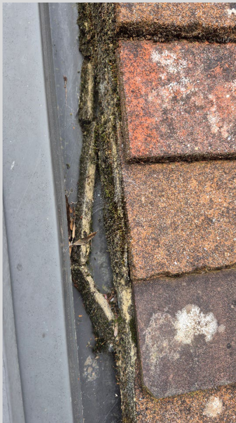
Image 12 - Secondary roof slope showing failing flashing around rooflights
