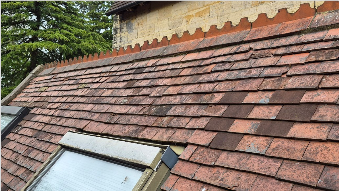
Image 11 - Secondary roof slope with evidence of slipped, delaminating and missing tiles
