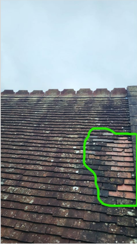
Image 9 – External view of North Kitchen roof with poor quality patch repair of tiles
