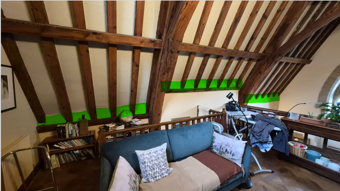
Image 5 - Internal view of North Kitchen roof with areas of water damage marked in green
