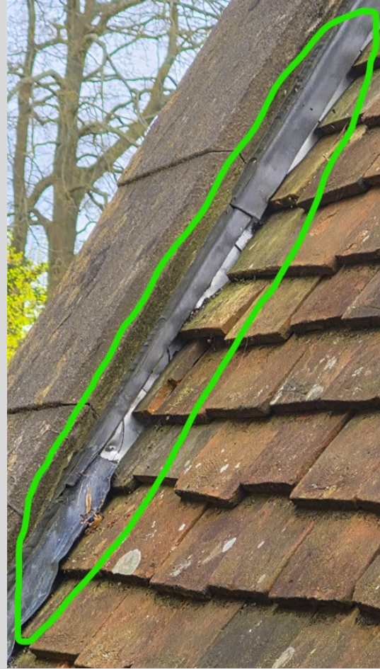
Image 10 – External view of North Kitchen roof with poor soaker and flashing repair evident
