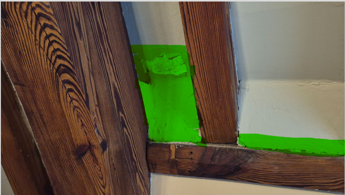
Image 6 - Close up image of water damage to internal face of North Kitchen roof – East Side
