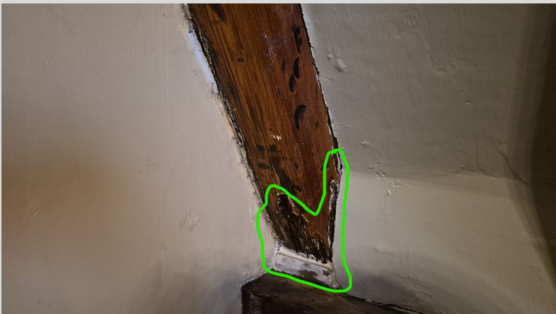
Image 8 - Close up image of water damage to main roof timber of North Kitchen roof
