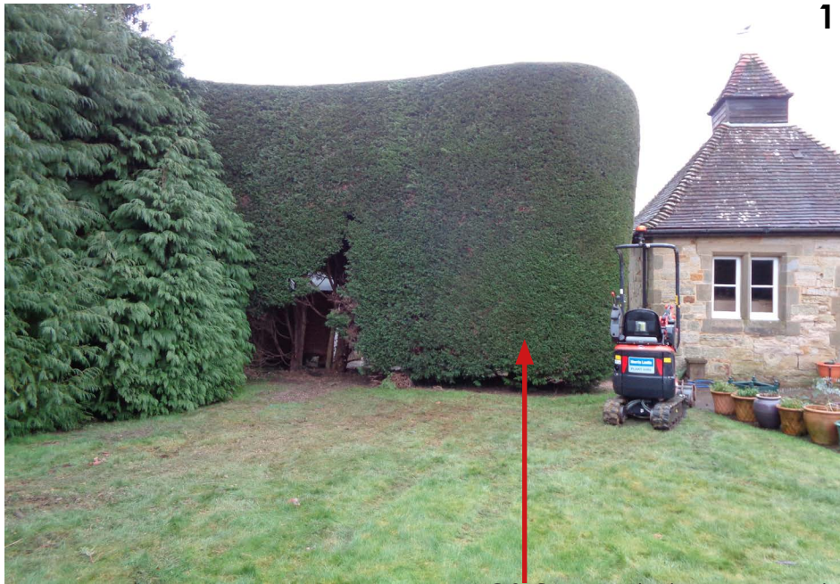
G8 Cypress to be removed.
