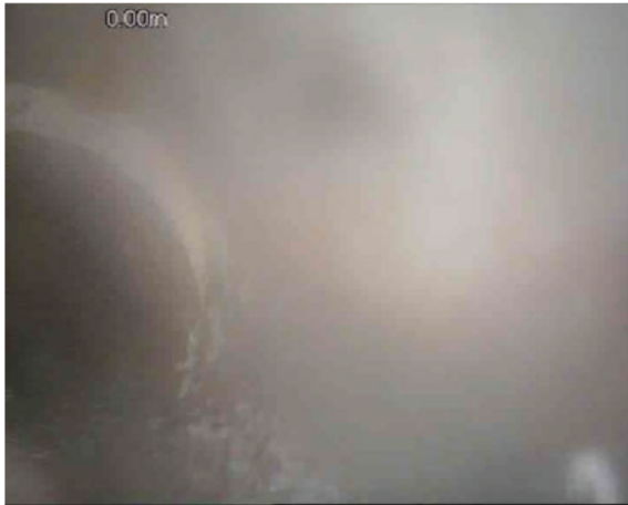
1, 00:00:11, 0.10 m Joint displaced, medium
