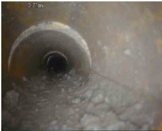
1, 00:00:19, 0.71 m Joint displaced, medium
