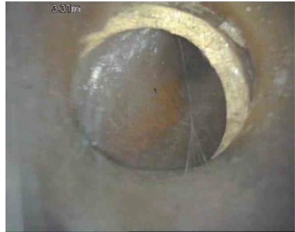
2, 00:00:22, 3.31 m Joint displaced, large
