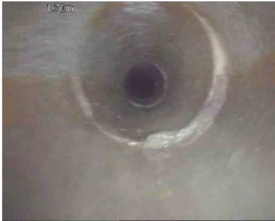
1, 00:00:19, 1.70 m Joint displaced, medium
