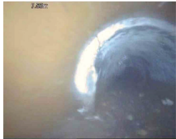
2, 00:00:39, 7.53 m Broken pipe at joint at 10 o'clock
