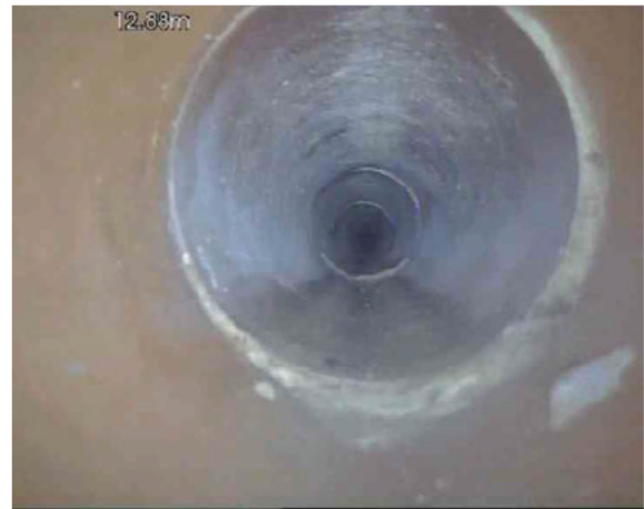
2, 00:00:52, 12.88 m Joint displaced, medium
