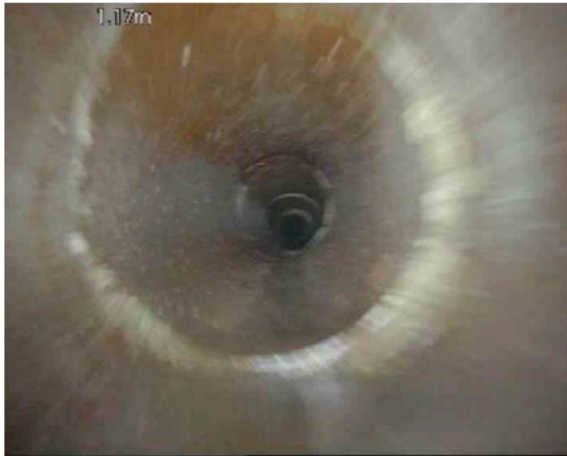
1, 00:00:18, 1.17 m Joint displaced, medium
