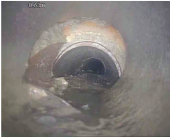
1, 00:00:19, 0.63 m Broken pipe from 8 o'clock to 11 o'clock
