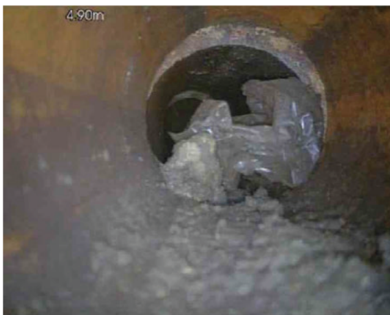
3, 00:00:41, 4.90 m Joint displaced, large
