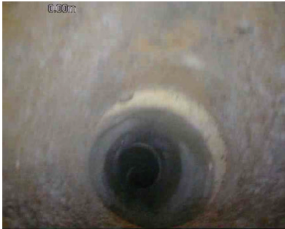
1, 00:00:11, 0.10 m Joint displaced, medium
