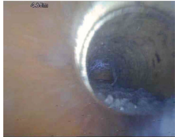
2, 00:00:32, 4.68 m Joint displaced, medium
