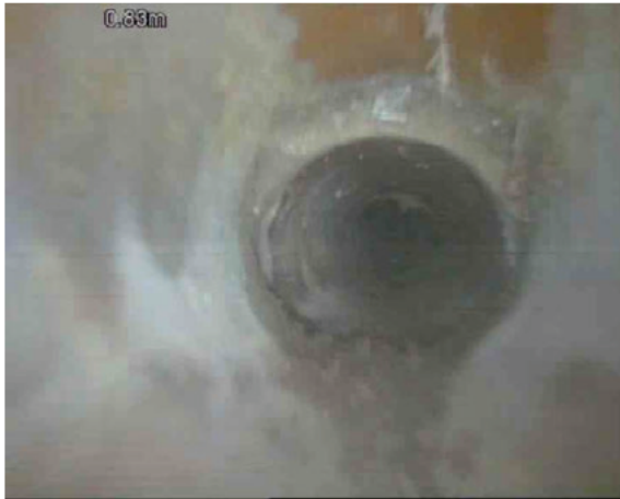
1, 00:00:15, 0.83 m Joint displaced, large
