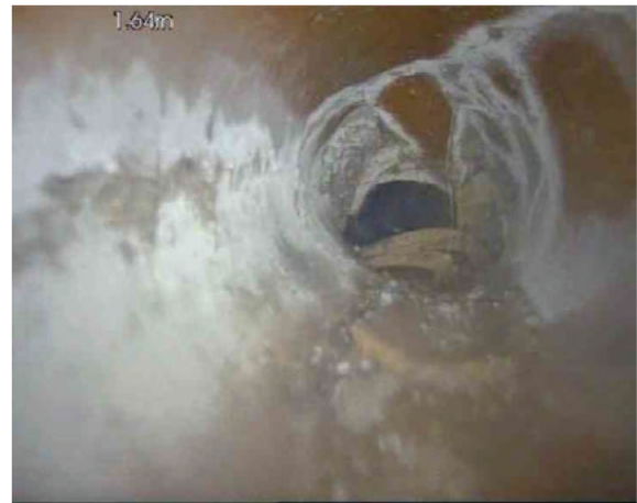
2, 00:00:16, 1.64 m Broken pipe from 5 o'clock to 7 o'clock
