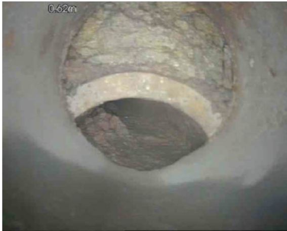
1, 00:00:14, 0.62 m Joint displaced, large
