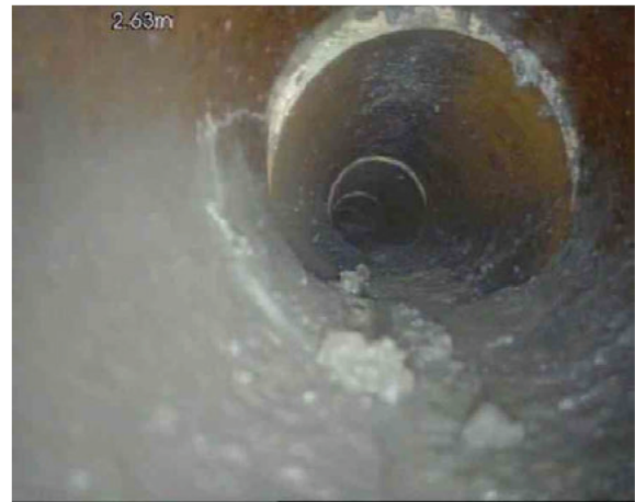
2, 00:00:27, 2.63 m Joint displaced, large
