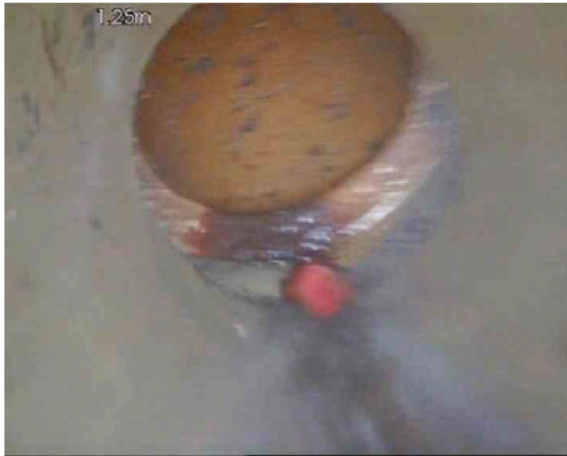
1, 00:00:21, 1.25 m Joint displaced, large
