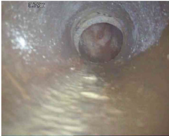
1, 00:00:15, 1.03 m Joint displaced, large
