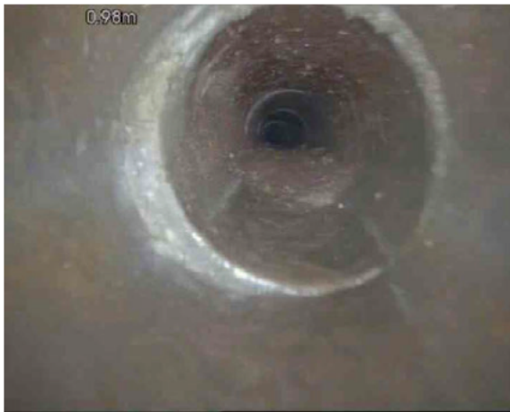
1, 00:00:15, 0.98 m Joint displaced, medium
