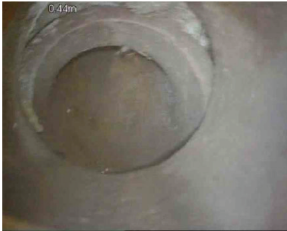
1, 00:00:15, 0.44 m Joint displaced, large
