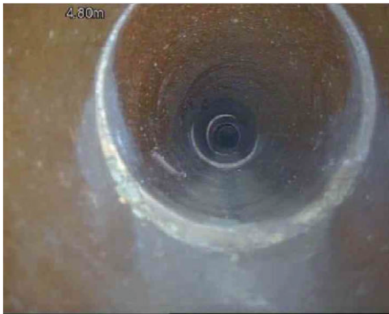
1, 00:00:25, 4.80 m Joint displaced, medium
