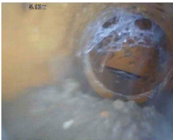
3, 00:00:34, 5.30 m Joint displaced, medium
