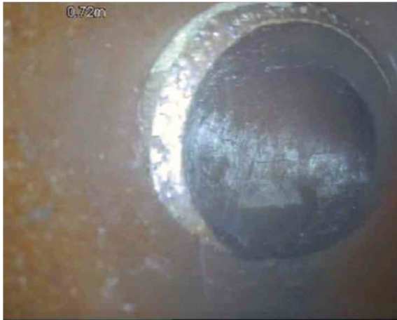
1, 00:00:15, 0.72 m Joint displaced, large
