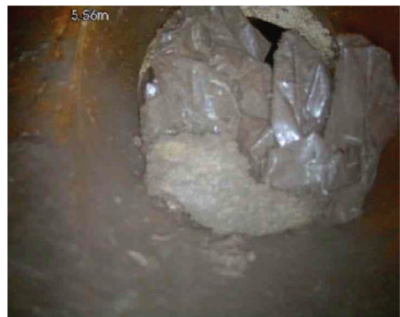
4, 00:01:02, 5.56 m Joint displaced, large
