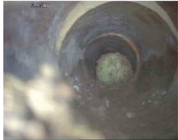
2, 00:00:28, 3.95 m Joint displaced, medium
