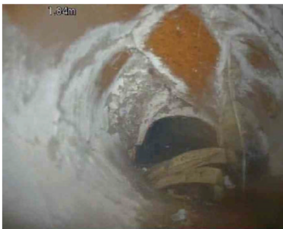
3, 00:00:17, 1.84 m Broken pipe from 9 o'clock to 4 o'clock
