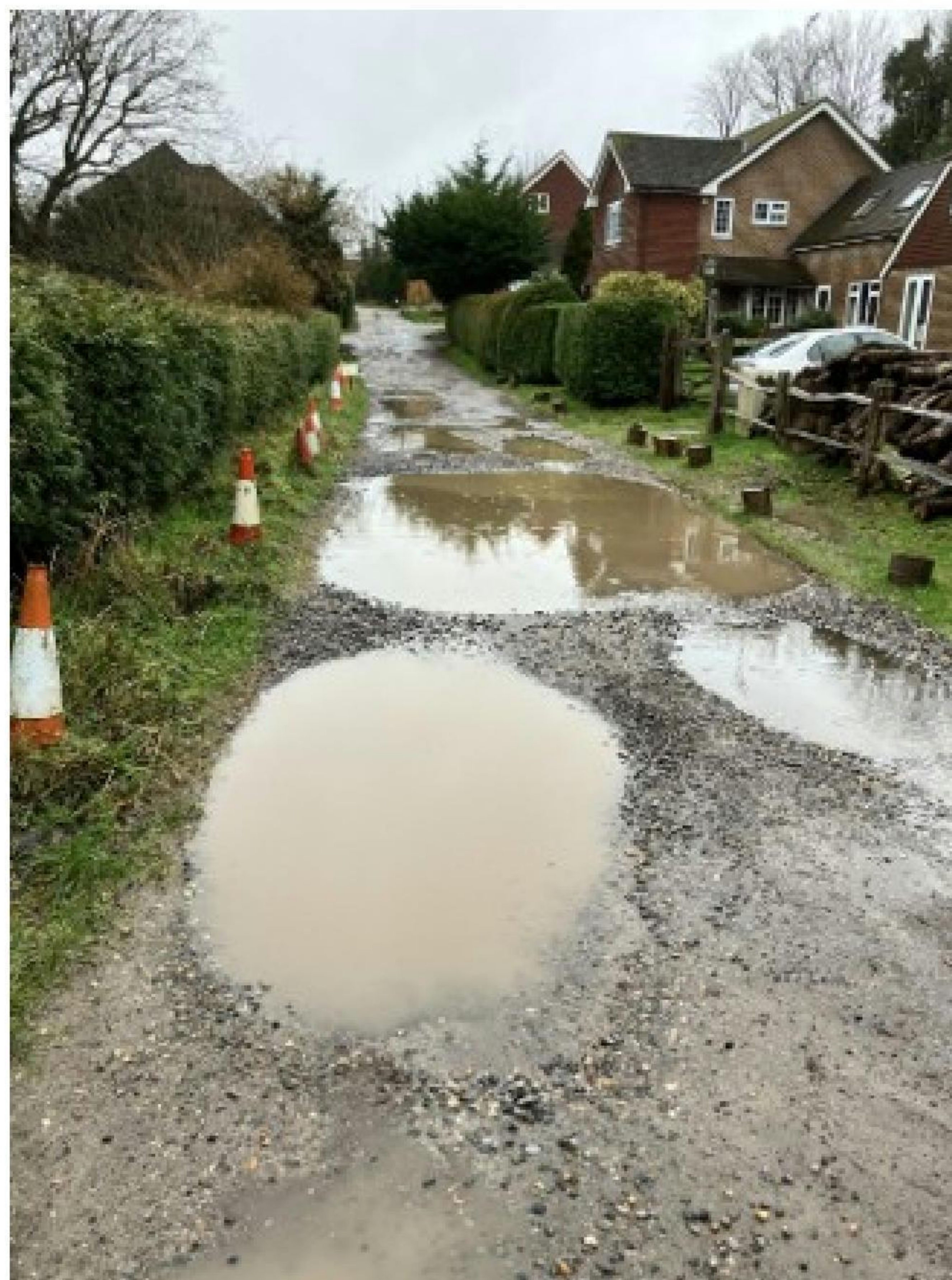
Photograph: the unadopted section of The Street between the site and the junction with Top Street, showing the potholed, waterlogged surface, the absence of any segregated footway or cycleway, and logs and cones placed to prevent use of the verges for passing.
