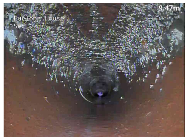
6, 00:01:13, 9.47 m Attached deposits, grease from 9 o'clock to 3 o'clock, 10% cross-sectional area loss, start
