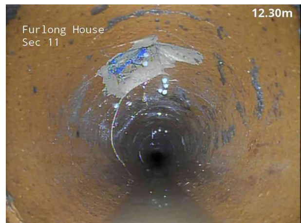
4, 00:01:31, 12.30 m Hole in drain or sewer at 11 o'clock
