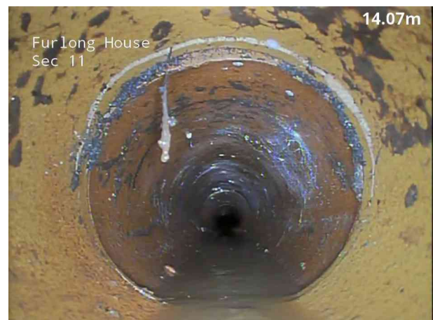
6, 00:01:44, 14.15 m Fracture, circumferential at joint from 9 o'clock to 3 o'clock
