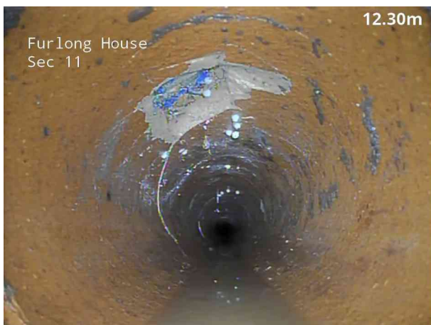
5, 00:01:31, 12.30 m Fracture, circumferential from 6 o'clock to 12 o'clock
