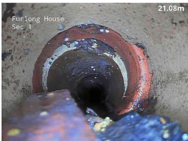
5, 00:03:57, 21.20 m Hole in drain or sewer from 11 o'clock to 1 o'clock
