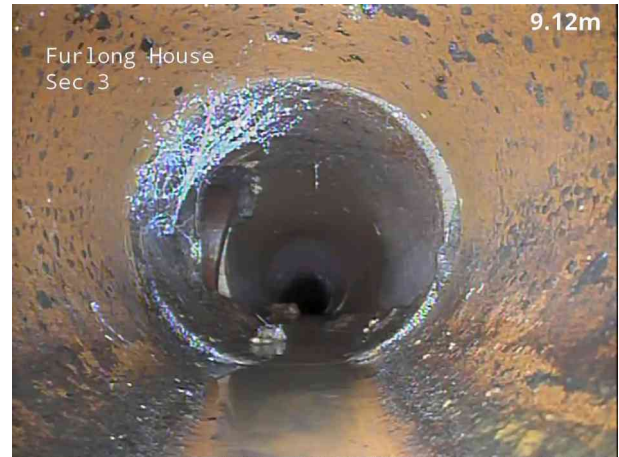
2, 00:01:08, 9.30 m Connection other than junction at 10 o'clock, 100mm dia
