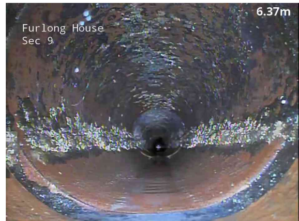
2, 00:00:50, 6.37 m Attached deposits, grease at 9 o'clock, 5% cross-sectional area loss, start
