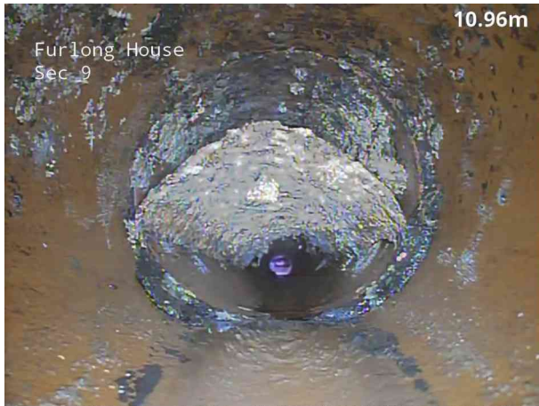
7, 00:01:30, 10.96 m Attached deposits, grease from 9 o'clock to 3 o'clock, 10% cross-sectional area loss, finish
