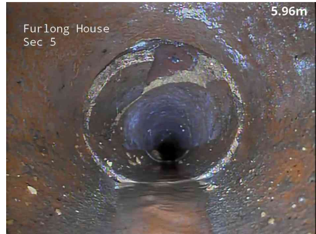
8, 00:00:57, 6.10 m Broken pipe at joint from 9 o'clock to 12 o'clock
