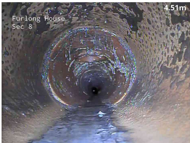
5, 00:00:52, 4.70 m Connection other than junction at 12 o'clock, 100mm dia
