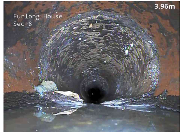
2, 00:00:41, 4.00 m Attached deposits, encrustation at joint from 4 o'clock to 8 o'clock, 5% cross-sectional area loss
