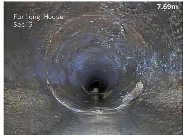
10, 00:01:21, 7.85 m Hole in drain or sewer from 4 o'clock to 5 o'clock
