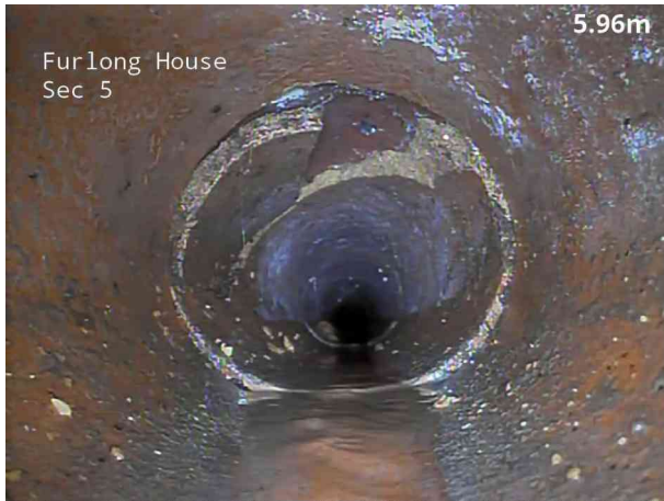
7, 00:00:57, 6.10 m Fracture, longitudinal at joint at 9 o'clock
