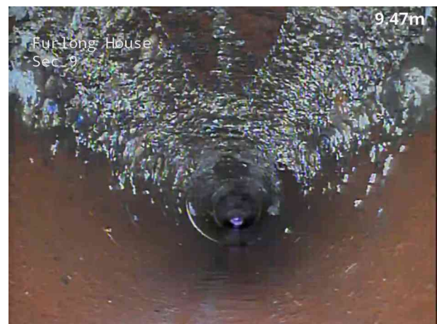
4, 00:01:13, 9.47 m Attached deposits, grease at 9 o'clock, 5% cross-sectional area loss, finish
