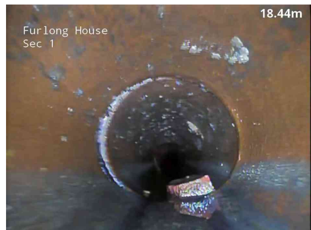
4, 00:03:19, 18.60 m Other obstacles, brick or masonry in invert at 5 o'clock, 5% cross-sectional area loss
