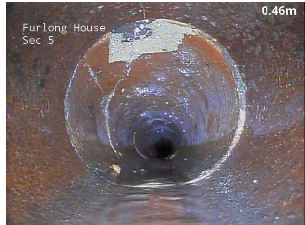
2, 00:00:12, 0.60 m Fracture, circumferential from 7 o'clock to 12 o'clock
