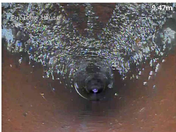
5, 00:01:13, 9.47 m Attached deposits, grease at 3 o'clock, 5% cross-sectional area loss, finish
