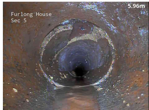
6, 00:00:57, 6.10 m Fracture, circumferential at joint from 9 o'clock to 1 o'clock
