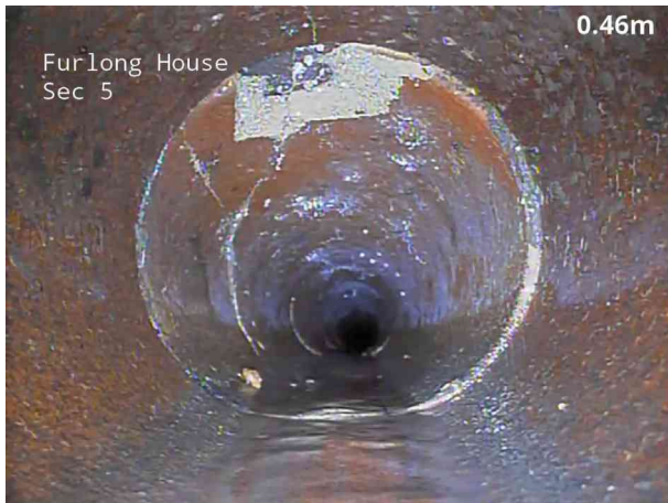
3, 00:00:12, 0.60 m Broken pipe at joint from 11 o'clock to 12 o'clock
