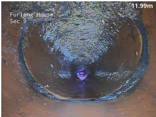
9, 00:01:42, 12.00 m Attached deposits, grease from 8 o'clock to 4 o'clock, 70% cross-sectional area loss, finish
