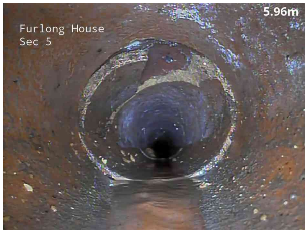
9, 00:00:57, 6.10 m Hole in drain or sewer from 12 o'clock to 1 o'clock
