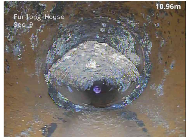
8, 00:01:30, 10.96 m Attached deposits, grease from 8 o'clock to 4 o'clock, 70% cross-sectional area loss, start
