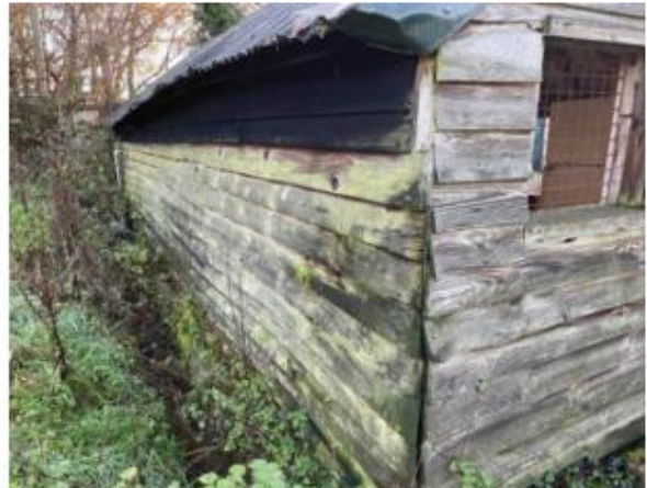
Warped weatherboarding at the western end of B2, with potential for crevice dwelling bats.
