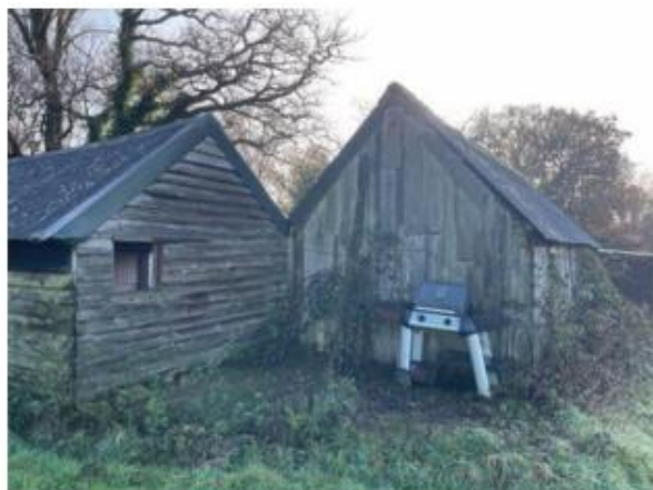
Northern gable end of B3 (right) and western gable end of B2 (left) with warped and rotten timber, creating potential crevice roosting features.
