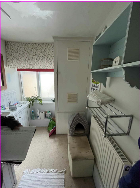
COTTAGE 5 BATHROOM PLANT CUPBOARD TO BE MADE BIGGER 800MM WIDE x 1000MM DEEP INTERNALLY TO MATCH COTTAGE 6 CUPBOARD..
