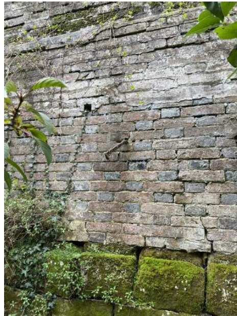
1.2 Multiple cracks in the brick wall above the stone base
