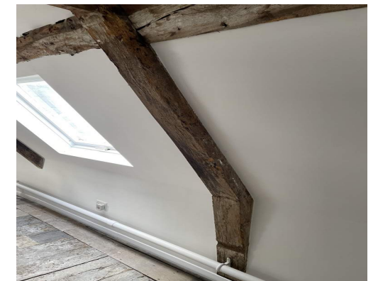
12 Full timber sections not visible, ideally during works all plaster soffits to be fully stripped to allow full inspection & treatment / repair of all primary framing
