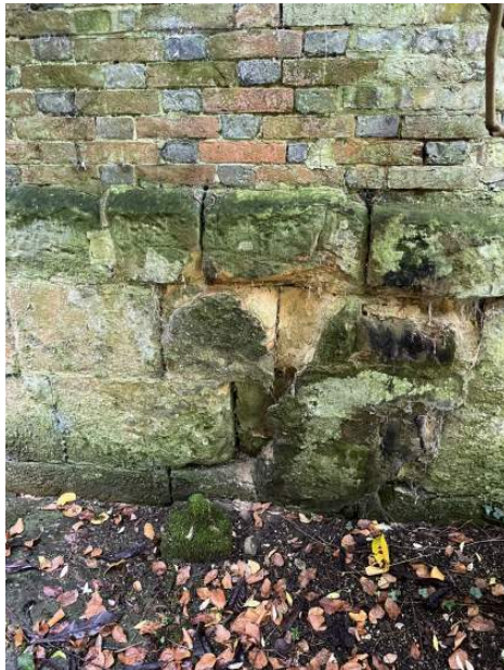
1.1 Severe defect in the stone base to the wall
