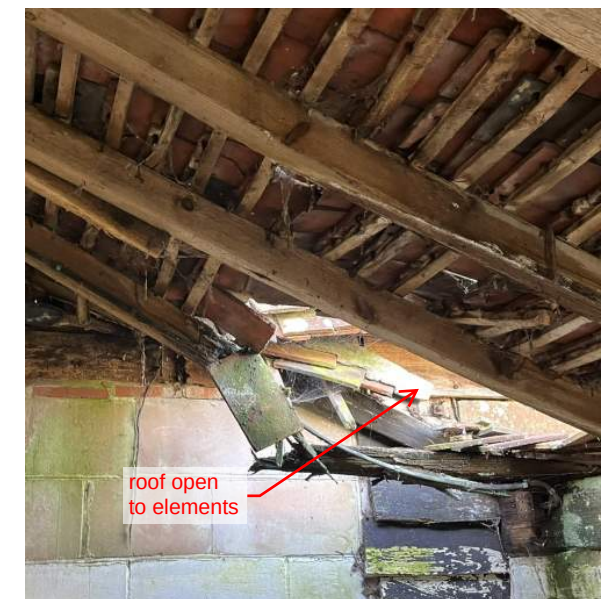
8 Failed rafter splices
