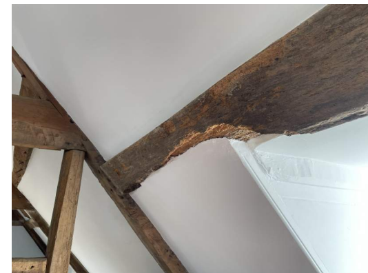
9 Areas of excessive decay and infestation particularly to sap wood sections of timbers detailed condition survey of attic timbers required by infestation specialist!
