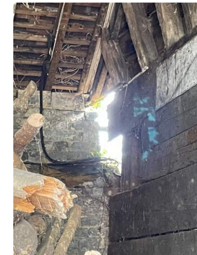
10 Hole in southern wall
