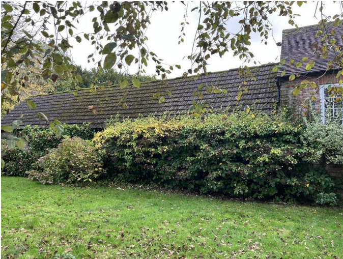
1 Northern elevation abutting stables, vegetation has grown excessively & is on brink of causing damage to roof eaves
