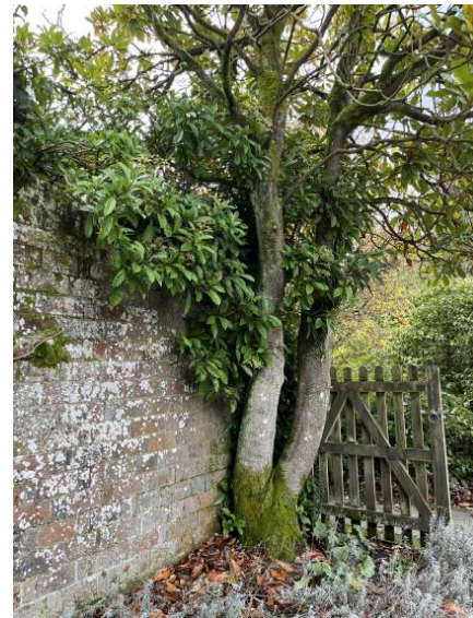
2 Laurel tree at wall end has grown against wall & is causing wall to lean
