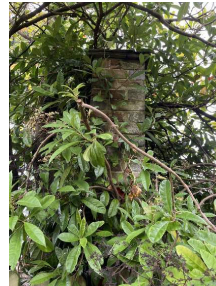
3 Visible excessive lean to wall end, not measured but approx 50-75mm over full height
