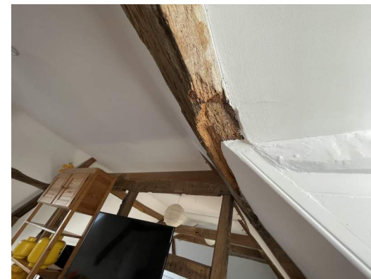
10 Underside view of severely depleted timber section
