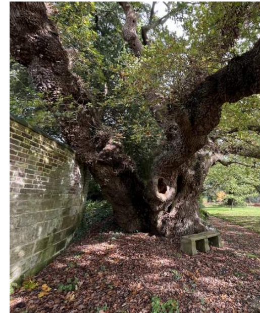
2.2 Visible distortion of wall by the oak tree
