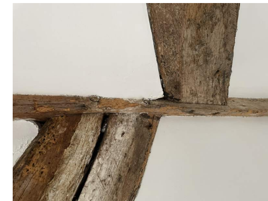
11 Illustrating varied surface conditions of timber elements, signs of natural drying splits, decay and infestation
