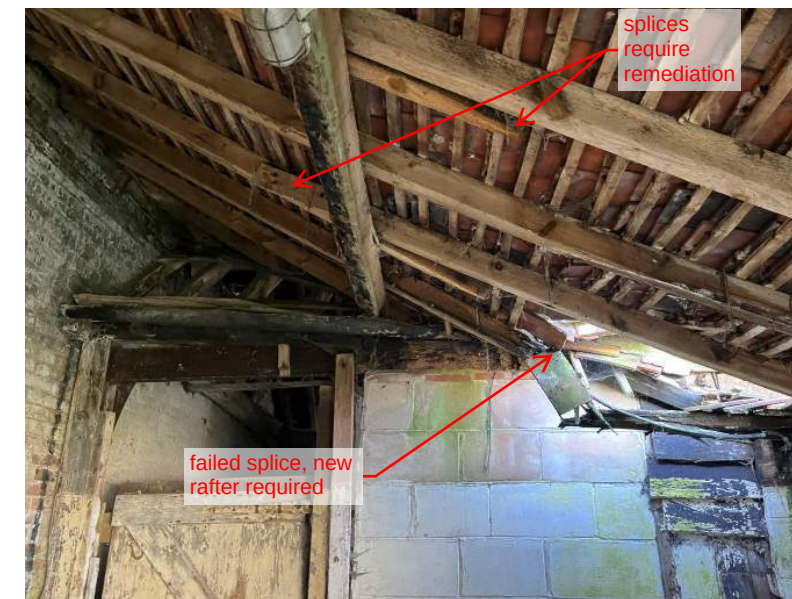
7 Wall to cow shed & collapsed roof
