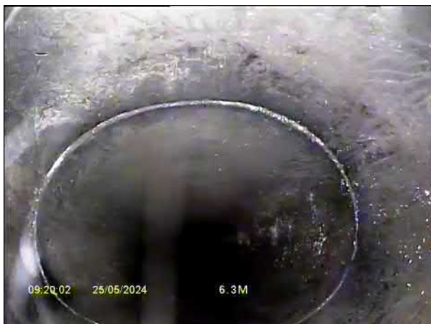
00:00:46, 6.30 m Deformed drain or sewer, 15%
