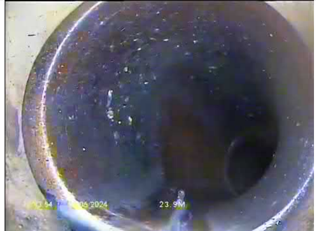
00:02:43, 5.00 m Line deviates right, full
