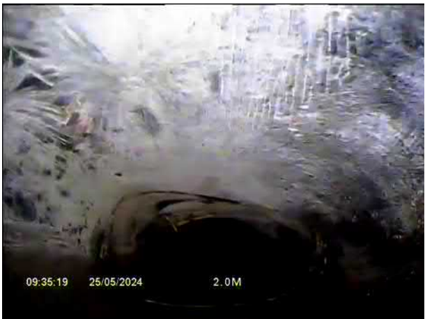
00:01:03, 2.10 m Deformed drain or sewer, 50%
