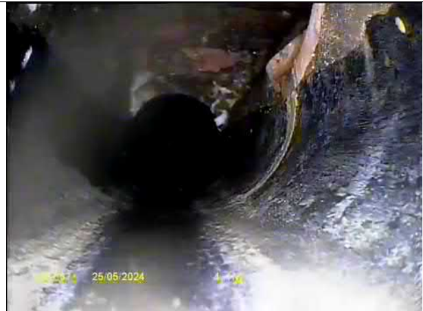
00:00:21, 4.40 m General remark, Manhole 04
