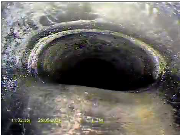
00:00:29, 1.20 m Deformed drain or sewer, 50%
