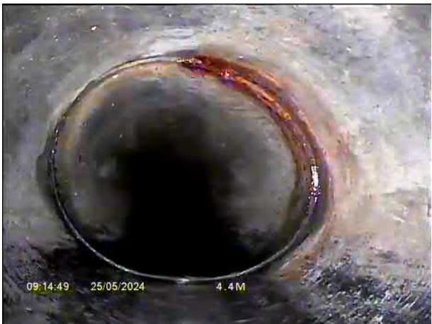
00:01:55, 4.40 m Deformed drain or sewer, 5%
