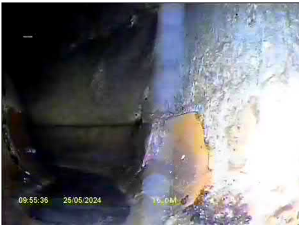
00:03:42, 16.00 m Finish manhole, MH02, the pipe is failing to discharge
