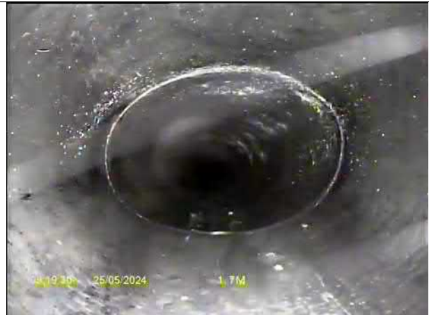
00:00:14, 1.70 m Deformed drain or sewer, 15%
