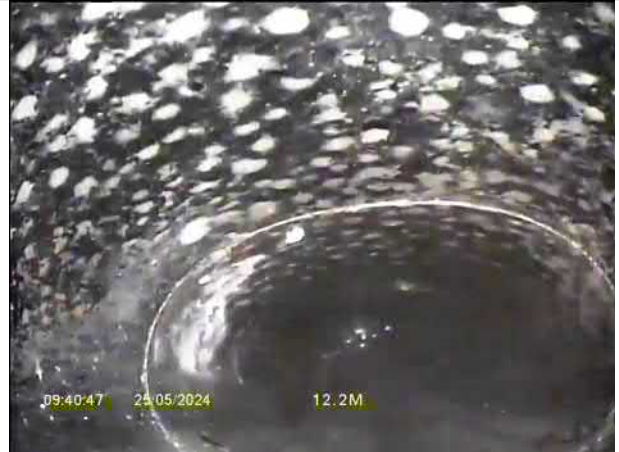
00:01:35, 12.20 m Deformed drain or sewer, 25%
