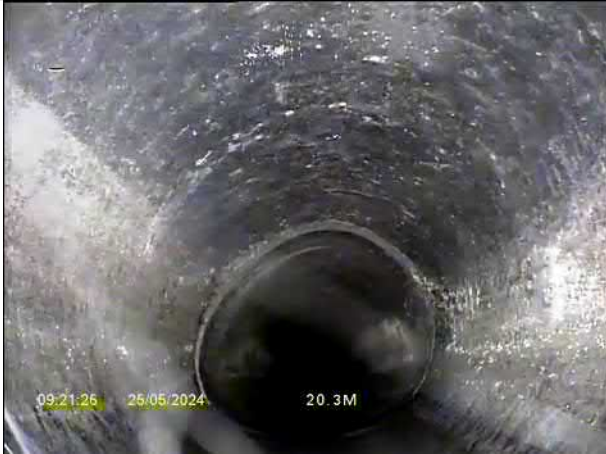
00:02:10, 20.00 m Deformed drain or sewer, 10%
