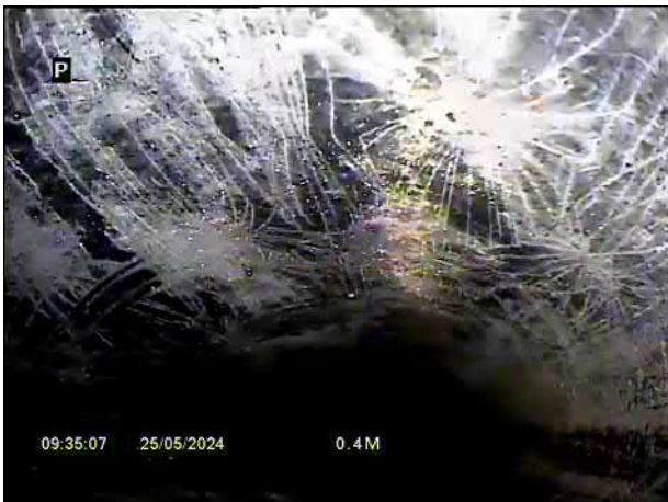
00:00:51, 0.40 m Deformed drain or sewer, 20%
