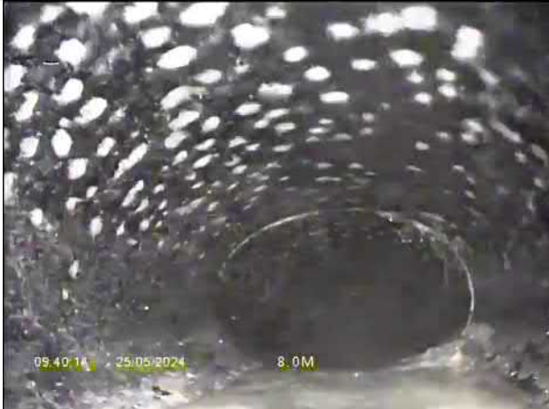
00:01:03, 8.00 m Deformed drain or sewer, 15%
