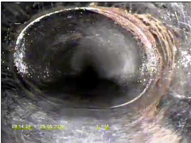
00:01:45, 1.90 m Deformed drain or sewer, 15%
