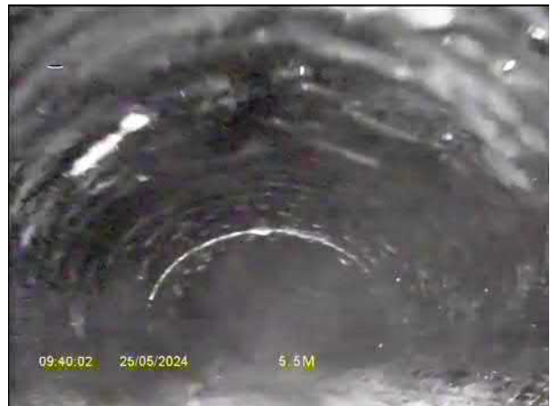
00:00:51, 5.50 m Deformed drain or sewer, 15%
