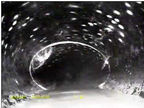
00:00:33, 3.30 m Deformed drain or sewer, 25%
