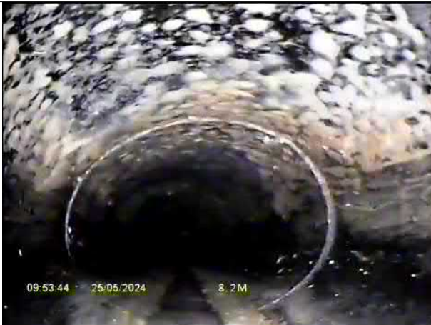
00:01:51, 8.20 m Deformed drain or sewer, 10%
