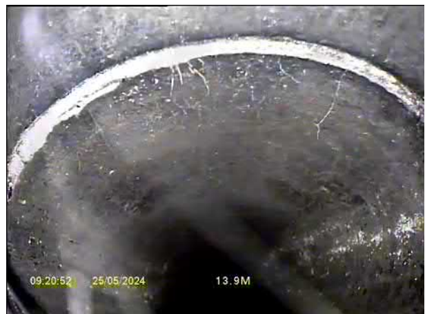
00:01:37, 14.00 m Deformed drain or sewer, 15%
