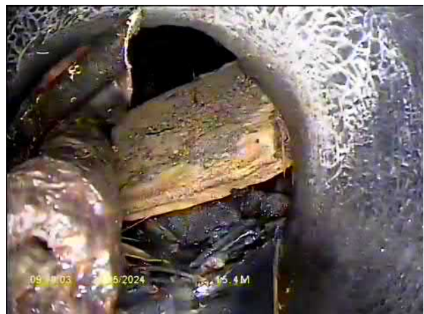
00:03:09, 15.40 m Other obstacles, 100% area loss, Manhole rendering and brickwork blocking channel
