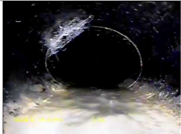
00:00:12, 0.50 m Deformed drain or sewer, 15%
