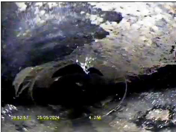
00:01:04, 4.20 m Deformed drain or sewer, 15%
