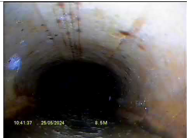
00:03:05, 8.50 m Deformed drain or sewer, 20%
