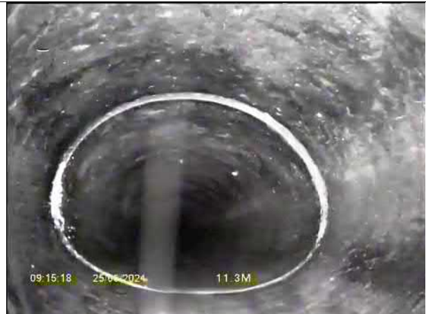
00:02:24, 11.30 m Deformed drain or sewer, 15%
