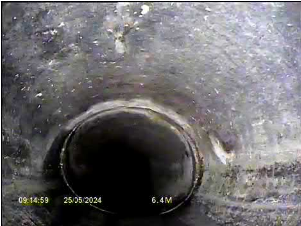
00:02:05, 6.40 m Deformed drain or sewer, 60%
