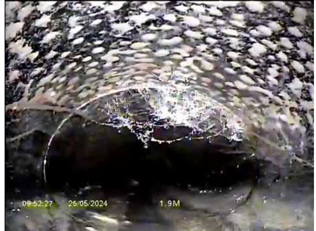
00:00:34, 2.00 m Deformed drain or sewer, 15%
