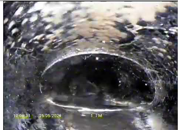
00:00:26, 1.70 m Deformed drain or sewer, 50%
