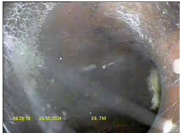
00:06:57, 38.70 m Line deviates right, full
