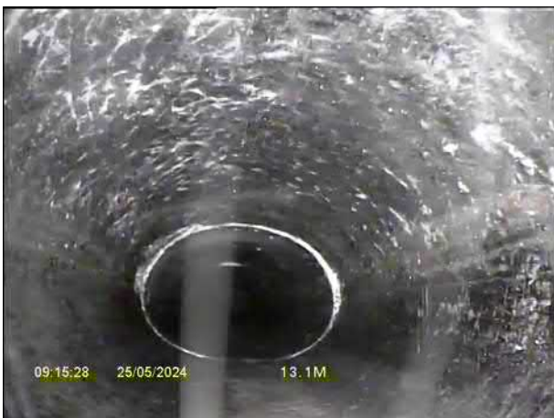
00:02:34, 13.50 m Deformed drain or sewer, 15%
