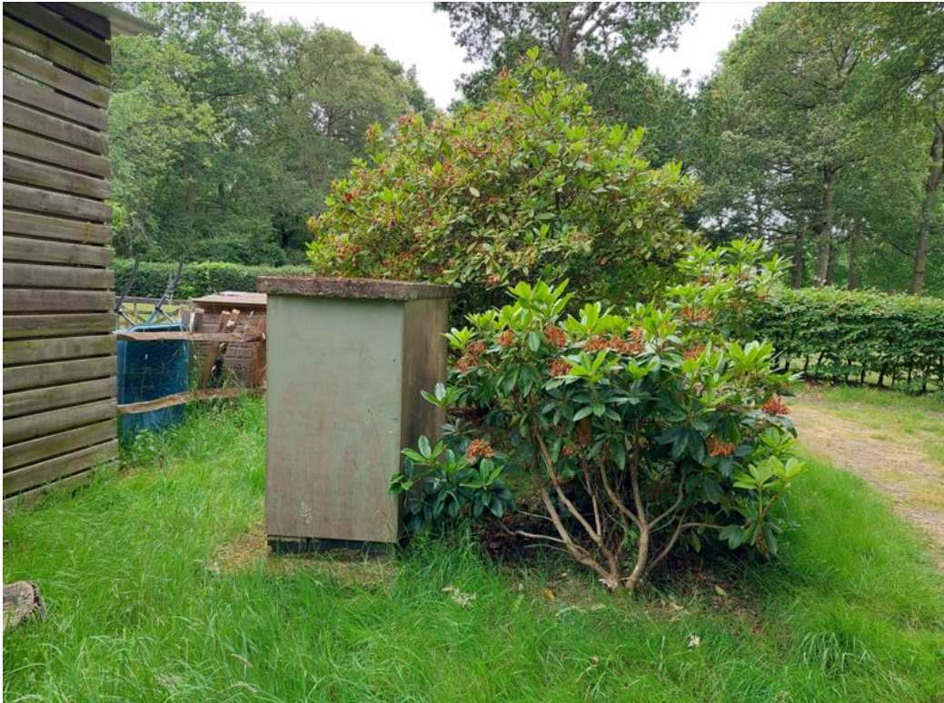
Photograph 7: Electrical intake cupboard to side of barn
