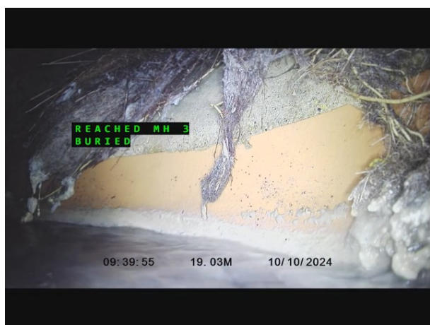
3, 00:00:51, 19.02 m Finish node, manhole, reference: MH3, Buried
