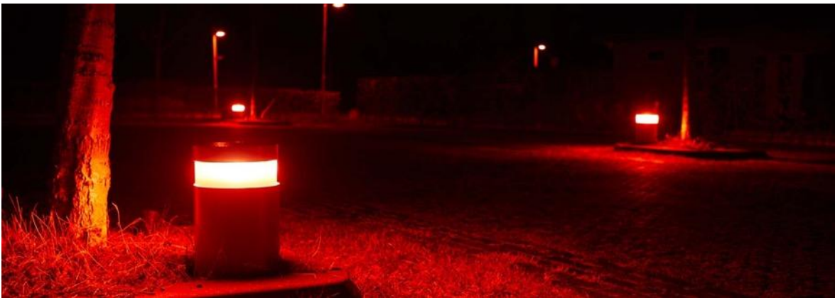
Figure 6: Example of low level bollard lighting
