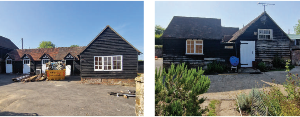
Examples of existing weatherboard condition
