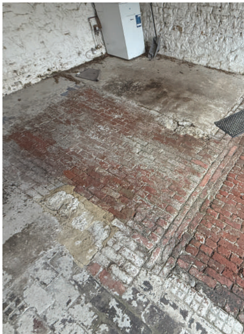
Example of Mid C19th floor to garage with later infill cement repairs among historic brick pavers
