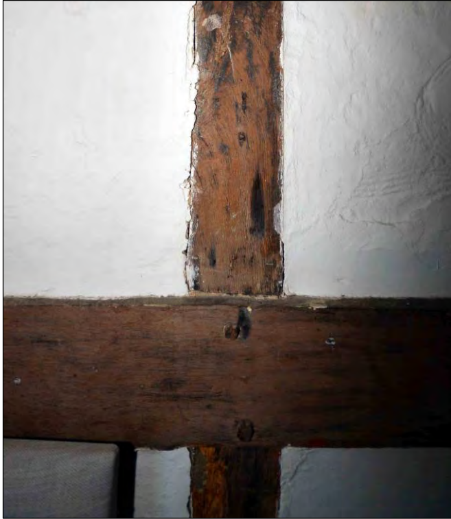
Plate 21: Two taper burns on the north side of the T4 truss in the first floor room
