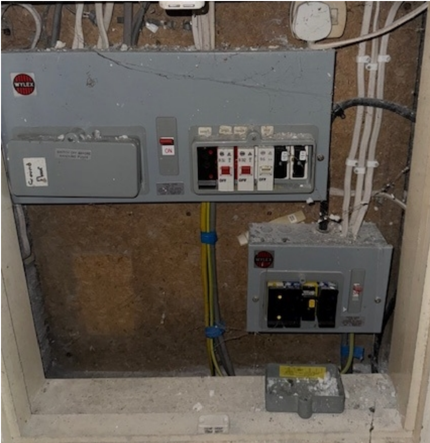
House fuse board.
