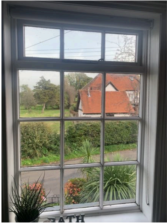
WINDOW B1: 1/4 X 3/4 Single glazed unit This is a bathroom window & gets very moldy & the paint peels off very year
