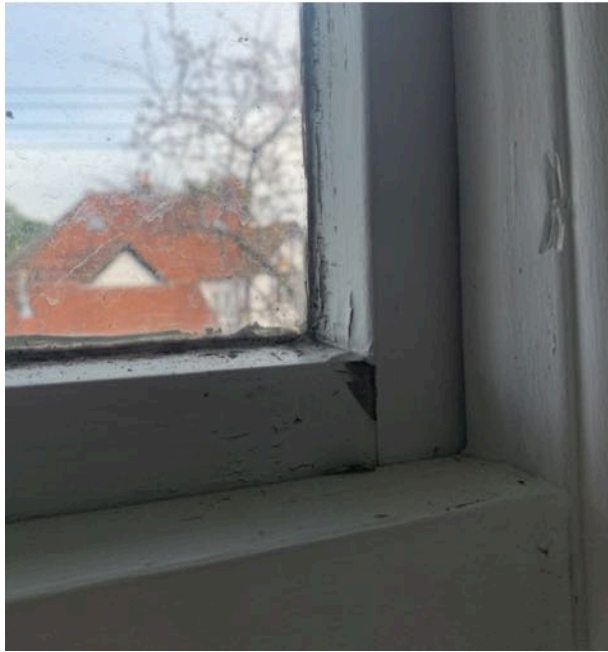
WINDOW B1: This window was renovated in 2021 and this is a detail picture which shows the paint already peeling off, due to condensation on the single glazed window
