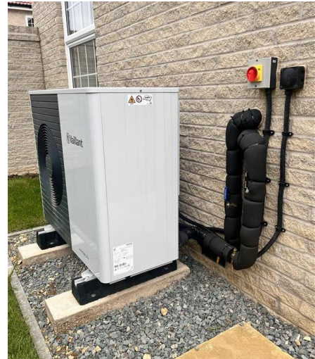
Picture: showing a ASHP connected to mains electric.
