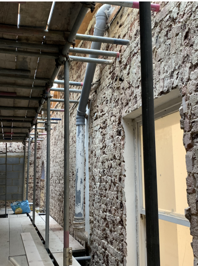
Second floor SVP 3 branch added into connection to take rainwater from roof, non original connection
