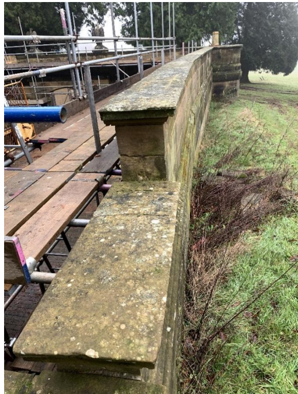
Wall bowed at high-level due to tree growth
