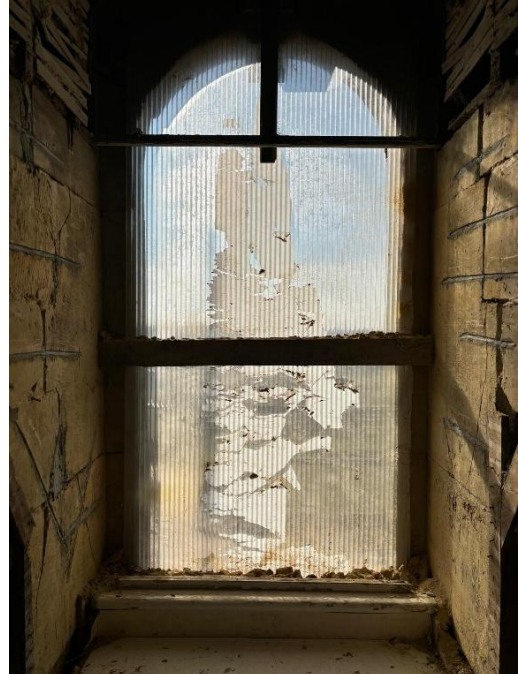
Type 2 – W2.06 with missing frame etc
