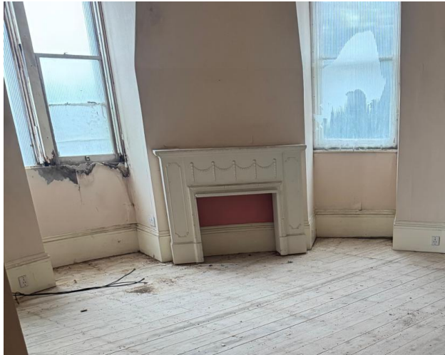
Type 1 - W2.08 with complete loss of original frames, cill, glazing and damage to central mullion
