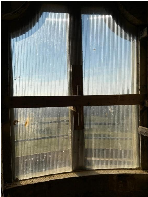
Type 1 – W2.04 with missing frame / glass
