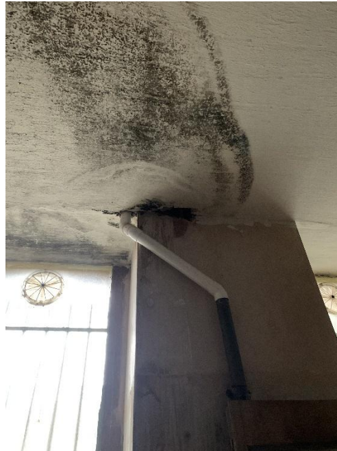
Modern, harmful pipework addition
