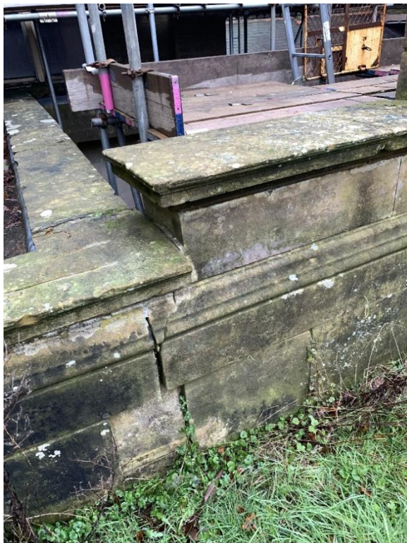
Cracked junction, courtyard wall and house
