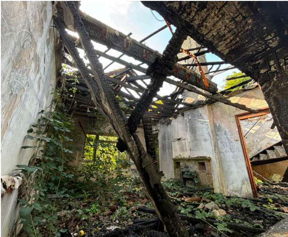
Existing dwelling, illustrating extent of fire damage
