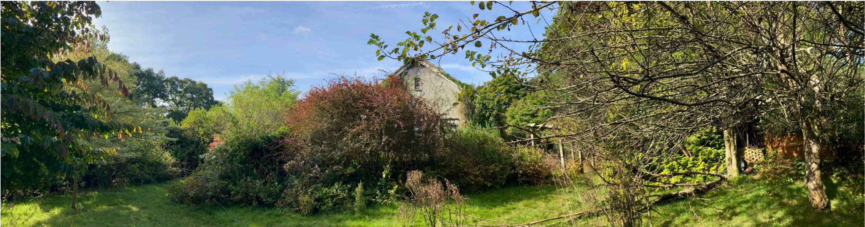
West elevation from rear garden obscured by overgrown vegetation.
