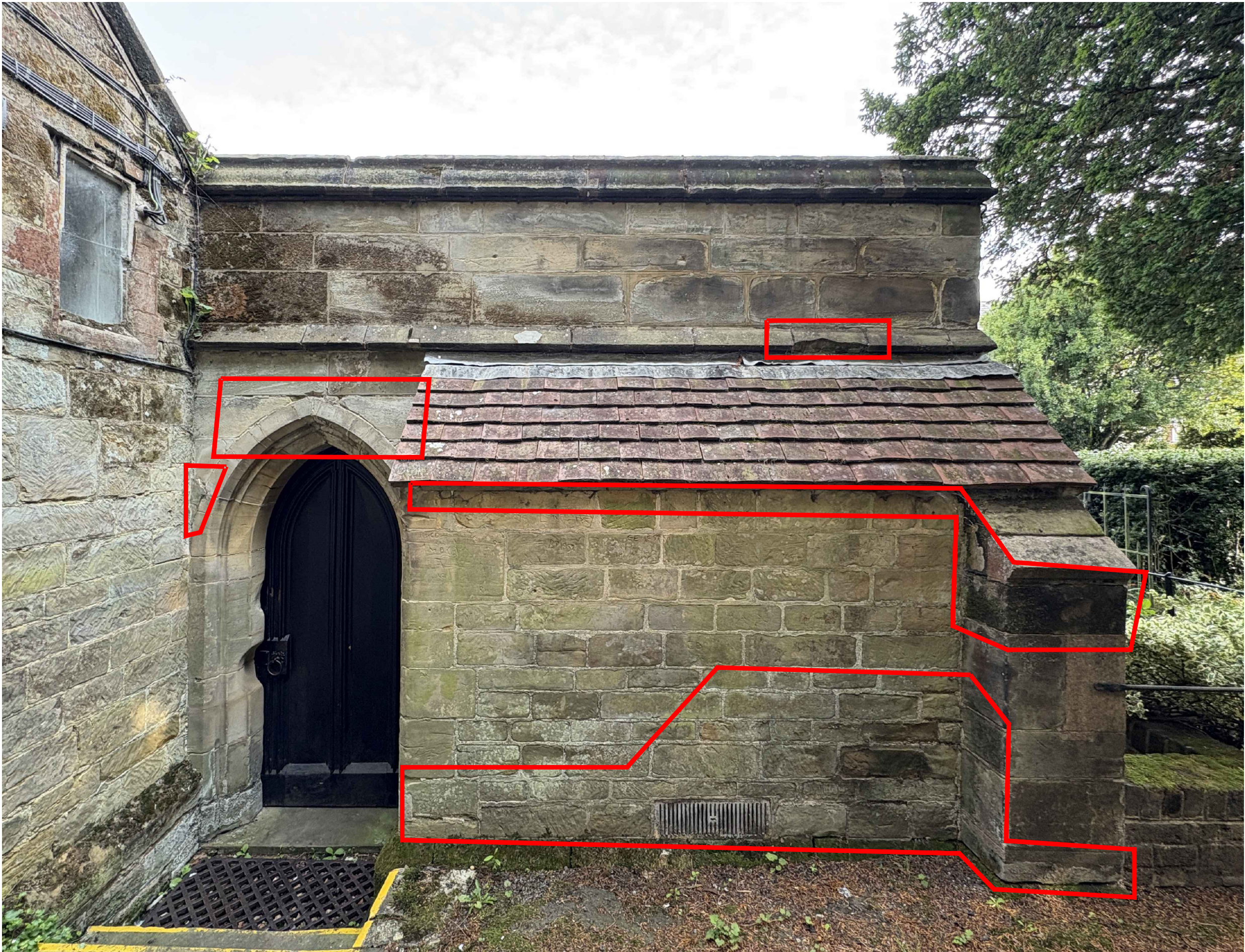
Stone work repairs hatched in colour.
