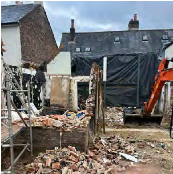
Bake house after its collapse during strip-out. Photograph provided by the Applicant.
