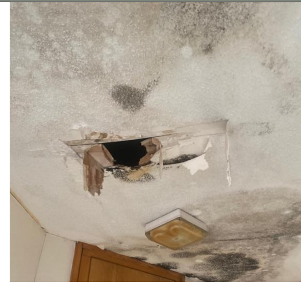
B1: hole in third storey ceiling leading to loft area
