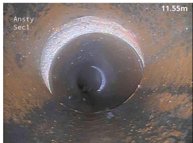
6, 00:00:52, 0.10 m Joint displaced, medium, start
