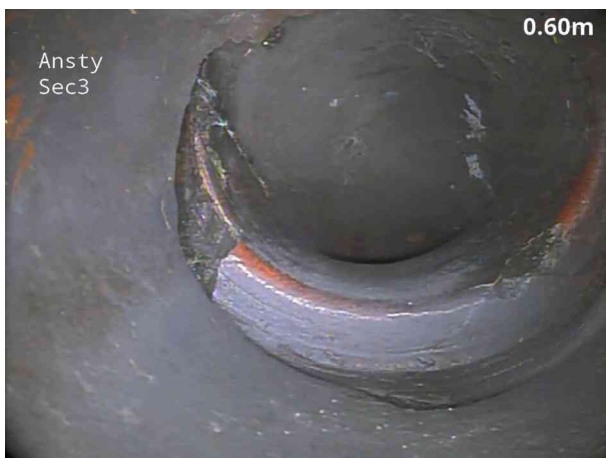
3, 00:00:20, 0.70 m Joint displaced, large
