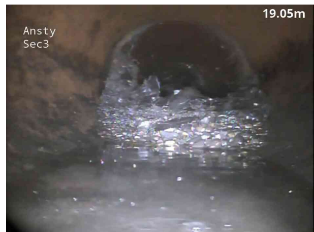
10, 00:02:11, 19.30 m Settled deposits, coarse, 60% cross-sectional area loss
