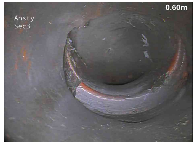
2, 00:00:20, 0.70 m Joint displaced, large
