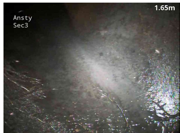
6, 00:00:43, 1.50 m Line deviates right, Junction onto carrier drain
