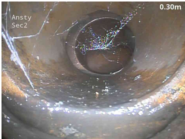
3, 00:00:13, 0.30 m Joint displaced, medium, start
