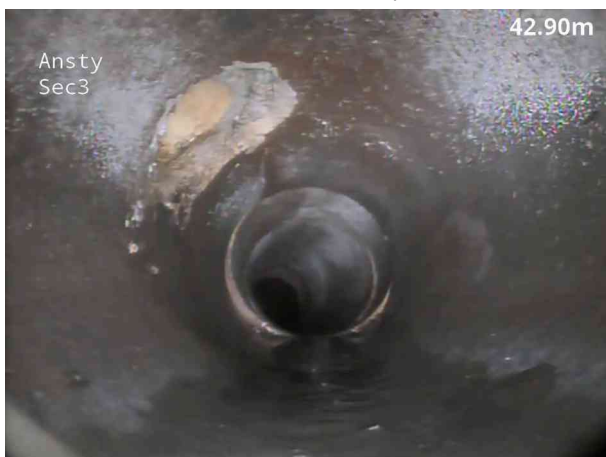
17, 00:03:51, 43.20 m Connection other than junction at 10 o'clock, 100mm dia
