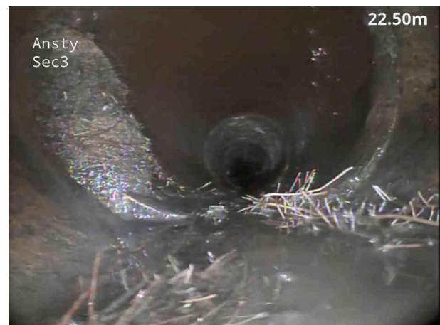
12, 00:02:33, 22.70 m Roots, mass at joint, 10% cross-sectional area loss
