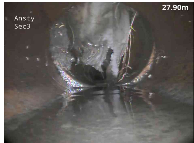
14, 00:02:50, 28.20 m Other obstacles at joint from 8 o'clock to 2 o'clock, 60% cross-sectional area loss, Upvc sheet
