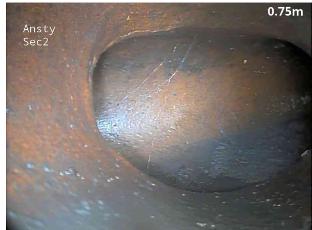
4, 00:00:22, 0.90 m Line deviates right, Junction onto carrier drain
