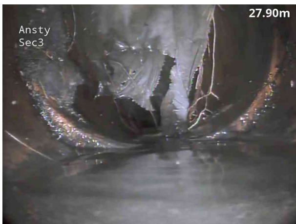
15, 00:02:50, 28.20 m Other obstacles at joint from 8 o'clock to 2 o'clock, 60% cross-sectional area loss, Upvc sheet
