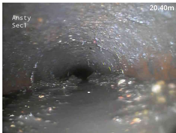
14, 00:02:27, 19.30 m Settled deposits, coarse, 60% cross-sectional area loss, start
