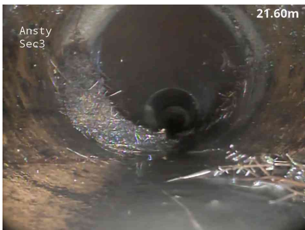
11, 00:02:30, 21.80 m Roots, mass at joint, 15% cross-sectional area loss
