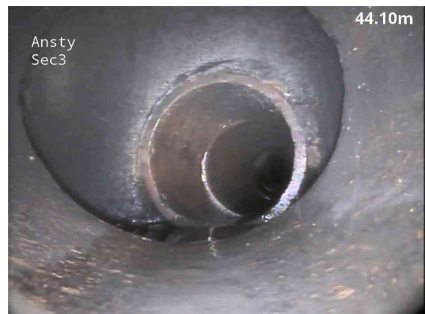
18, 00:04:07, 44.40 m Finish node, catchpit, reference: CP3, Buried
