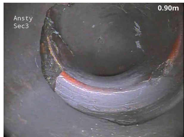
4, 00:00:29, 0.80 m Line deviates down
