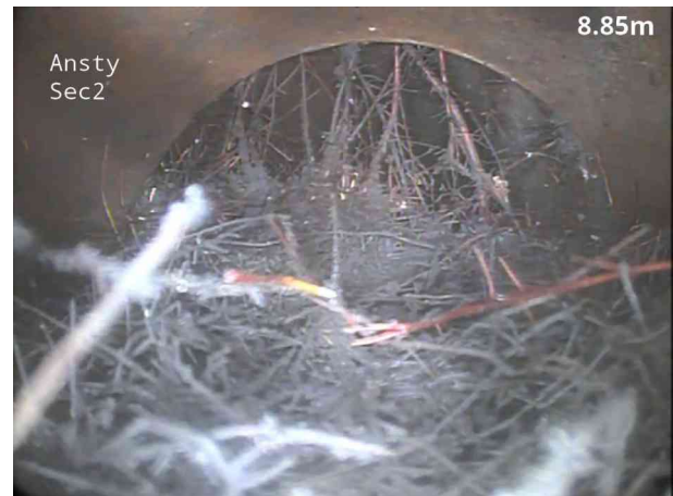
14, 00:01:35, 8.70 m Roots, mass, 70% cross-sectional area loss
