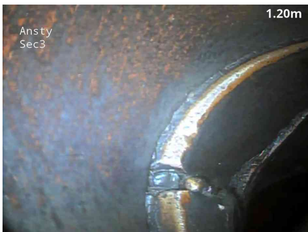
5, 00:00:39, 1.30 m Broken pipe at joint from 6 o'clock to 12 o'clock
