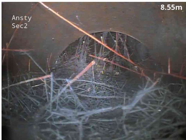
13, 00:01:35, 8.70 m Roots, mass, 70% cross-sectional area loss
