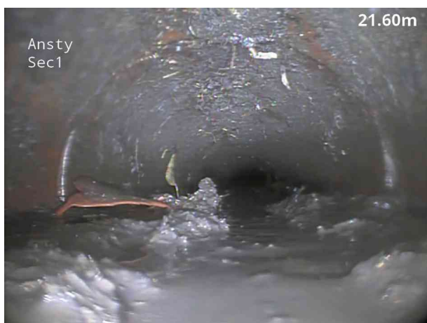
15, 00:02:56, 21.60 m Settled deposits, coarse, 50% cross-sectional area loss, change
