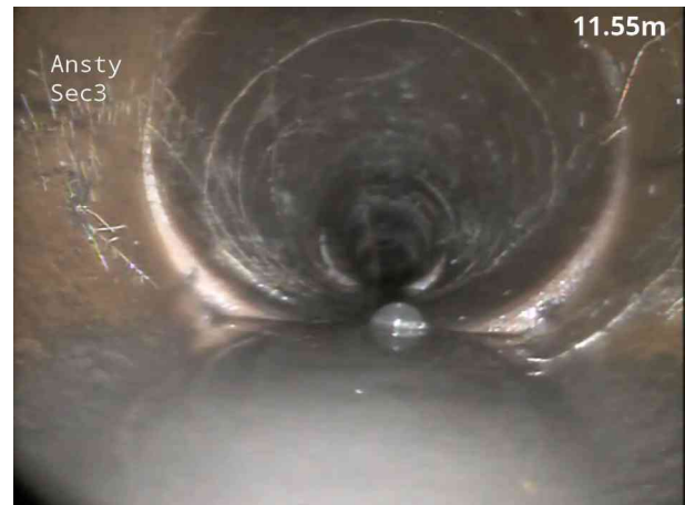
8, 00:01:38, 11.80 m Fracture, circumferential at joint from 12 o'clock to 12 o'clock
