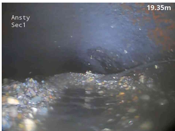
13, 00:02:27, 19.30 m Settled deposits, coarse, 60% cross-sectional area loss, start
