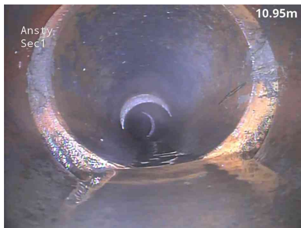
8, 00:01:42, 11.10 m Roots, fine at joint
