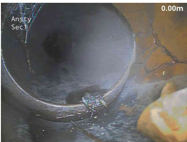
5, 00:00:52, 0.10 m Joint displaced, medium, start
