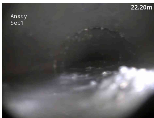
16, 00:03:42, 22.20 m Settled deposits, coarse, 60% cross-sectional area loss, change
