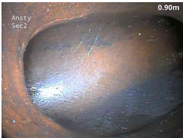
5, 00:00:22, 0.90 m Line deviates right, Junction onto carrier drain
