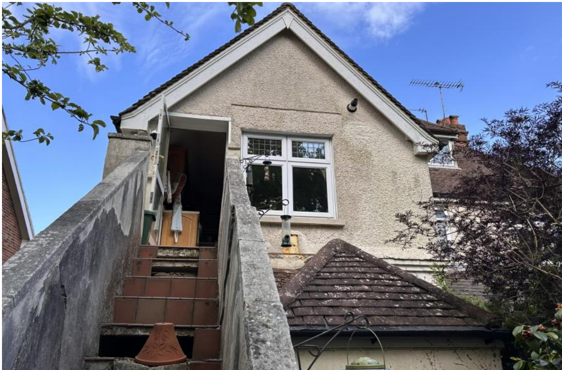
View at rear of dilapidated staircase requiring replacement.
