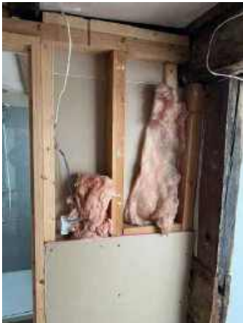
Poor quality bathroom wall build up exposed before demolition
