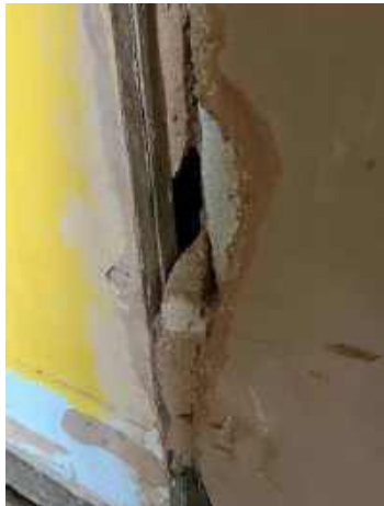
Poor quality bathroom wall before demolition
