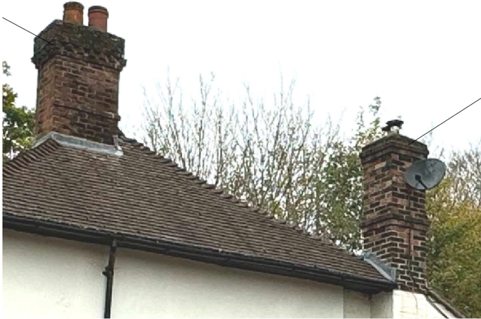
Chimney 3 to be repointed (left) and the unaffected chimney (right).
