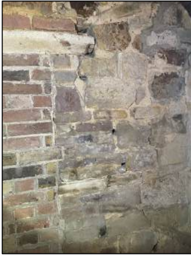
Photograph 5: Damage to the stonework internally within building B1.
