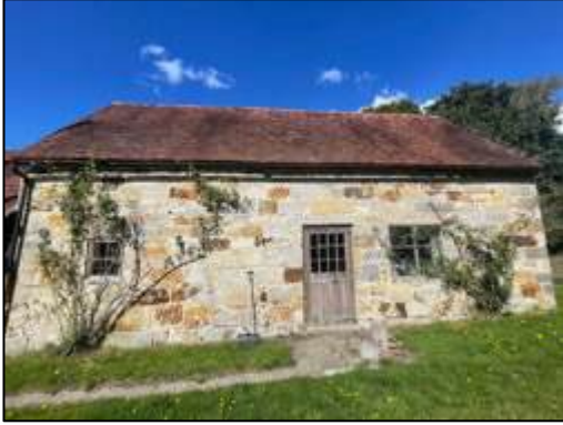
Photograph 1: The eastern elevation of building B1. Photograph showing the lifted roof tiles here.
