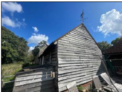
Photograph 9: The south-western elevation of building B2. Photograph showing the lifted weatherboarding here.
