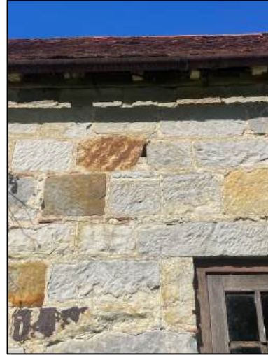
Photograph 2: Gaps in the external stonework of building B1.
