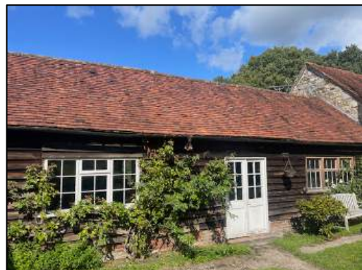
Photograph 10: The eastern elevation of building B2. Photograph showing the lifted tiles here.
