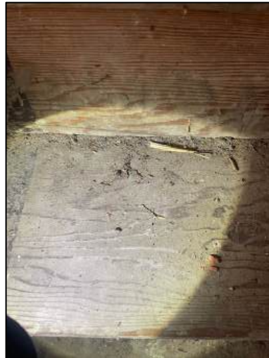
Photograph 8: One of the bat droppings within building B1.
