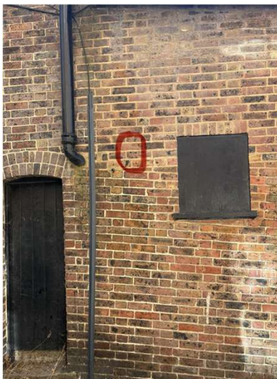
Images showing location of new extract grill for mechanical ventilation from gents' toilet facilities in basement
