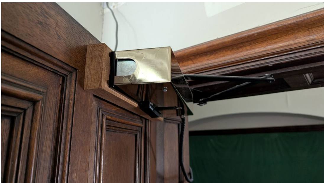
-5 Below, closer to be removed.
