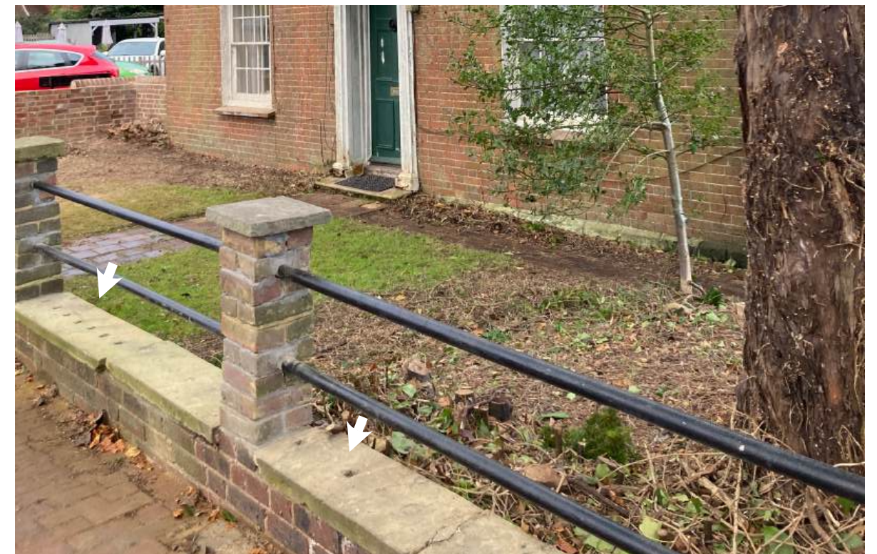
Scaffolding posts to be replaced with traditional metal railing. Arrows pointing holes from removed railings.
