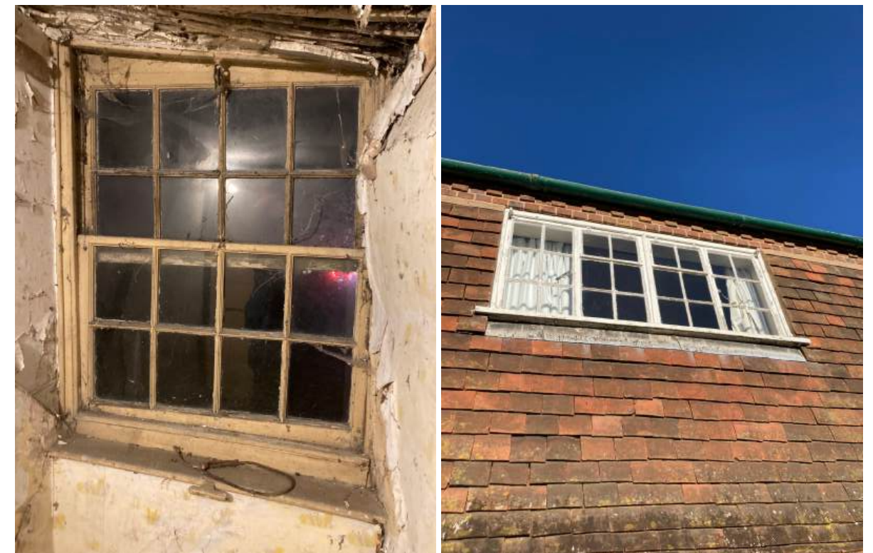
Example of decayed historic window to be replaced (left) and 1950s window to be replaced (right).
