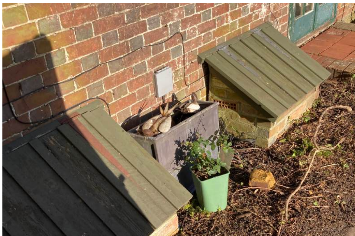
Modern cellar windows' covers to be replaced.
