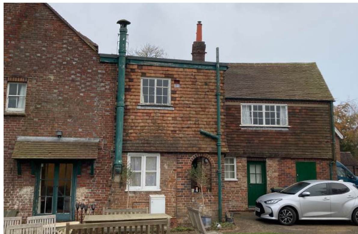
Modern pipes and soil vent pipes to be rationalised and intrinalised.
