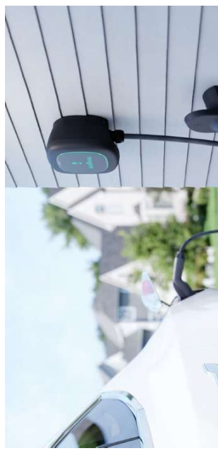
Electric Vehicle Charging Point
