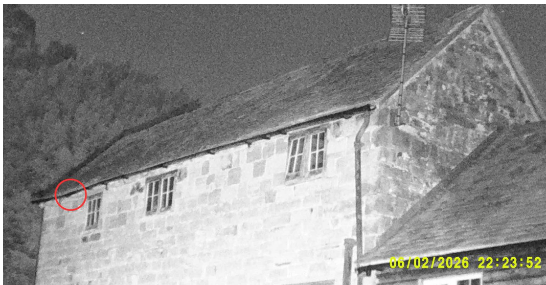
Image No. 08 – B1, northwest aspect. Re-entry at 22:24 on 02/06/2026 between guttering and eaves. Access point circled in red.
