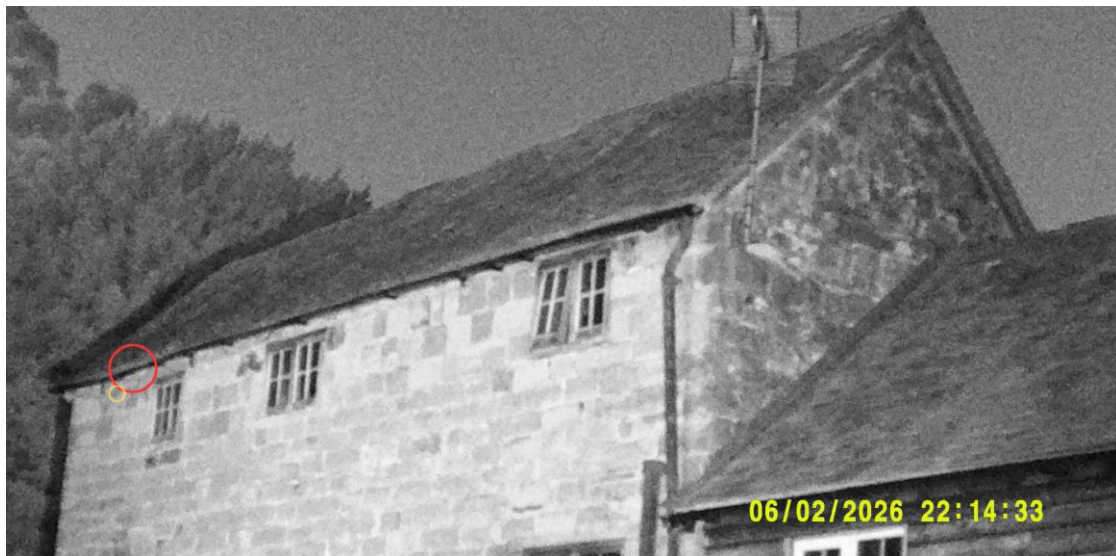
Image No. 06 – B1, northwest aspect. Re-entry at 22:15 on 02/06/2026 between guttering and eaves. Access point circled in red, bat visible faintly, circled in yellow to the left.
