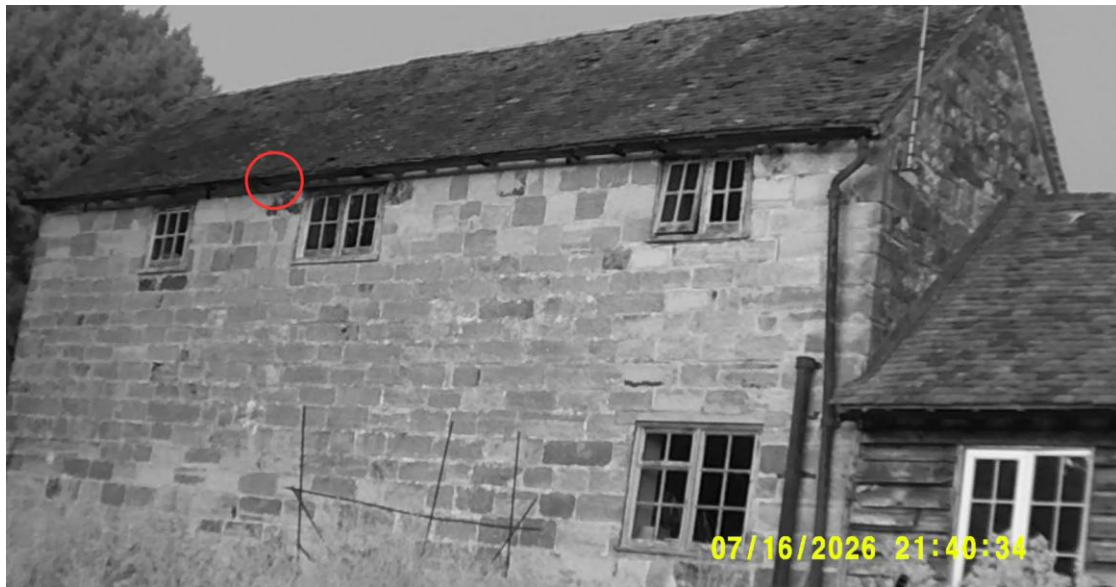
Image No. 09 – B1, northwest aspect. Emergence at 21:40 on 16/07/2026 between guttering and eaves. Emergence point circled in red.
