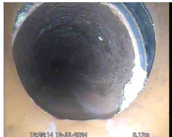
MH5X_f2943572-daea-4cc0-b643-02d9ae5cd5ee_20240725_094641_129.jpg, 00:00:44, 0.17 m Material changes to vitrified clay
