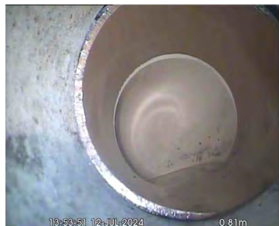
SVPX_6dc84003-04ba-4f4b-a2bc-ade636d85d44_20240725_095258_153.jpg, 00:00:43, 0.81 m Material changes to polyvinyl chloride
