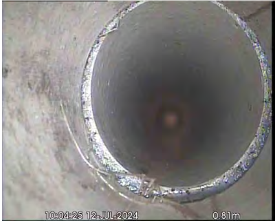
GULLYX_be408751-b267-4dcb-87b2-47920da53df0_20240725_090226_317.jpg, 00:01:01, 0.81 m Joint displaced, medium
