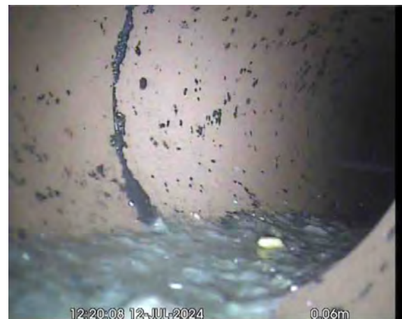
CAPPED OFFX_962b07f7-60c1-43c4-ba8a-1193030da8e6_20240725_094225_233.jpg, 00:00:42, 0.06 m Settled deposits, fine, 5% cross-sectional area loss
