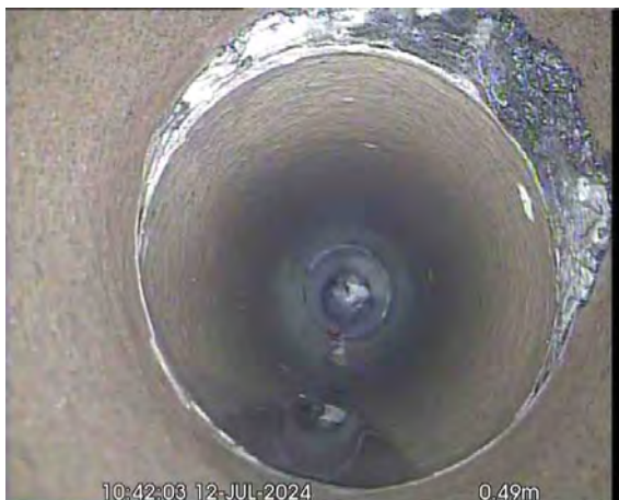
REDUNDANTX_0df9520d-4cc8-45ca-b8b9-6ea8c8cc1138_20 240725_091130_965.jpg, 00:00:34, 0.49 m Joint displaced, large
