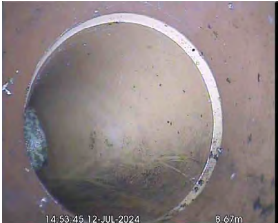
RWDPX_9497cd0e-eee7-4c16-afb8-0b0c38f1904e_20240725_101729_175.jpg, 00:01:16, 8.67 m Line deviates left
