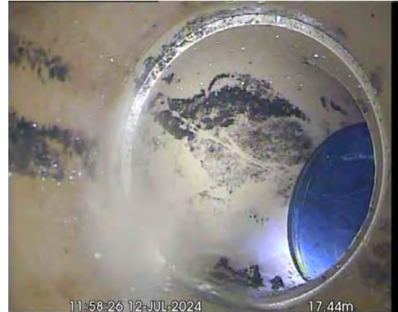
MH2X_ecbc01d4-5401-430c-a4cc-4e8128ef4209_20240725_093238_853.jpg, 00:02:20, 17.44 m Line deviates right
