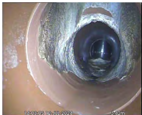
GULLYX_299e09be-81f4-44b5-a1cc-c1a653637af6_20240725_101416_847.jpg, 00:01:16, 3.42 m Junction at 12 o'clock, diameter: 110mm, W/C
