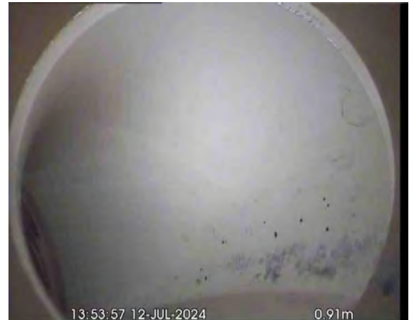
SVPX_1a7c91c5-7811-4395-aac0-3828833b4982_20240725_095342_984.jpg, 00:00:49, 0.91 m Line deviates left
