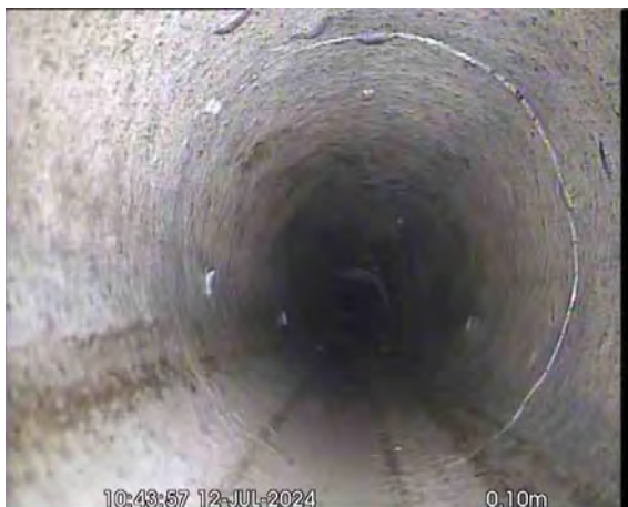
MH6X_d2fe370d-baf2-4429-b37e-bc117d0a8e8e_20240725_091559_829.jpg, 00:00:23, 0.10 m Fracture, circumferential from 11 o'clock to 5 o'clock
