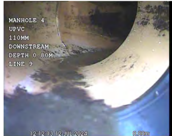
MH4X_b15f3203-8bce-4b3c-aea4-e017105a17a3_20240725_093849_179.jpg, 00:00:26, 0.00 m Water level, 0% of the vertical dimension
