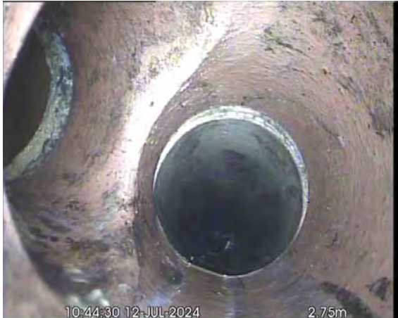
MH6X_522ba9e2-59fb-4d77-8b4f-20a3a199147f_20240725_092301_286.jpg, 00:00:56, 2.75 m Junction at 9 o'clock, diameter: 100mm, UNKNOWN
