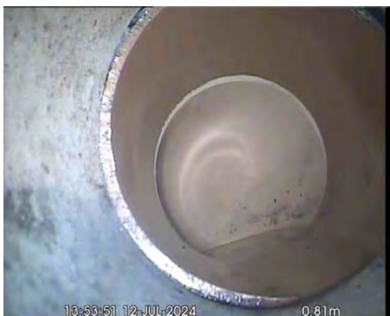
SVPX_6126ff3a-8feb-42cf-b4a8-289a35627abd_20240725_095243_344.jpg, 00:00:43, 0.81 m Joint displaced, medium
