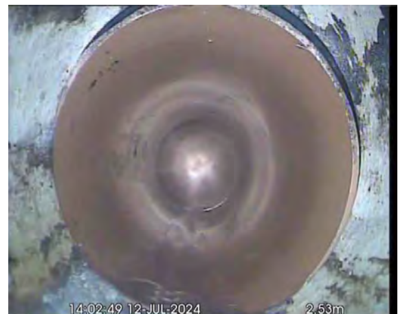
GULLYX_a0d2ed5e-7b7e-4ae5-a077-94c7952a4929_20240725_101329_585.jpg, 00:01:00, 2.53 m Joint displaced, medium
