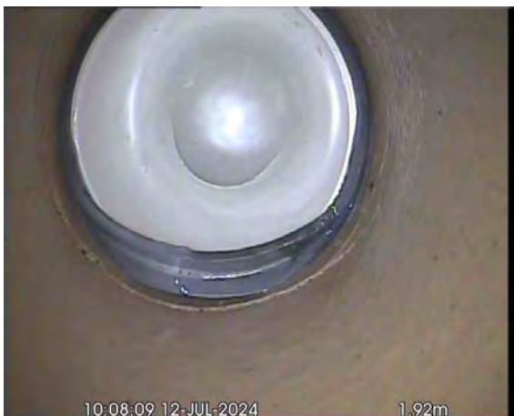
W_CX_140950e0-f4b9-4fa9-b1b6-8f3dc2314eb6_20240725_090748_590.jpg, 00:01:01, 1.92 m Crack, circumferential at joint from 12 o'clock to 12 o'clock
