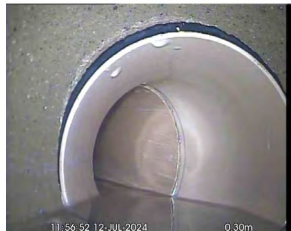
MH2X_9e3848a9-2aef-4403-9dc0-06a55e9cccf0_20240725_092609_653.jpg, 00:00:56, 0.30 m Joint displaced, medium
