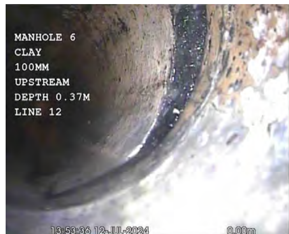
SVPX_74d44b96-72da-442c-8602-c87605640ac0_20240725_095222_464.jpg, 00:00:28, 0.00 m Water level, 0% of the vertical dimension
