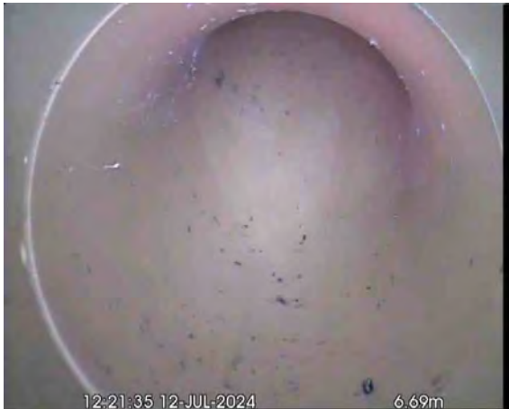
CAPPED OFFX_7b6014f4-cab8-4f12-9a9c-6eb32ef0d8f9_20240725_09 4246_571.jpg, 00:02:08, 6.69 m Line deviates up, REST BEND
