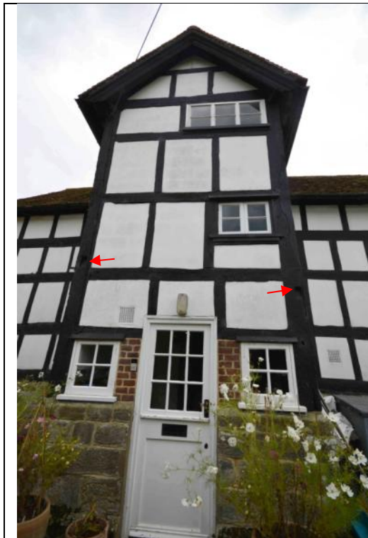
Plate 37: Scotches cut into the two principal posts on the north side of the tower during the under-building of the timber frame (arrows)
