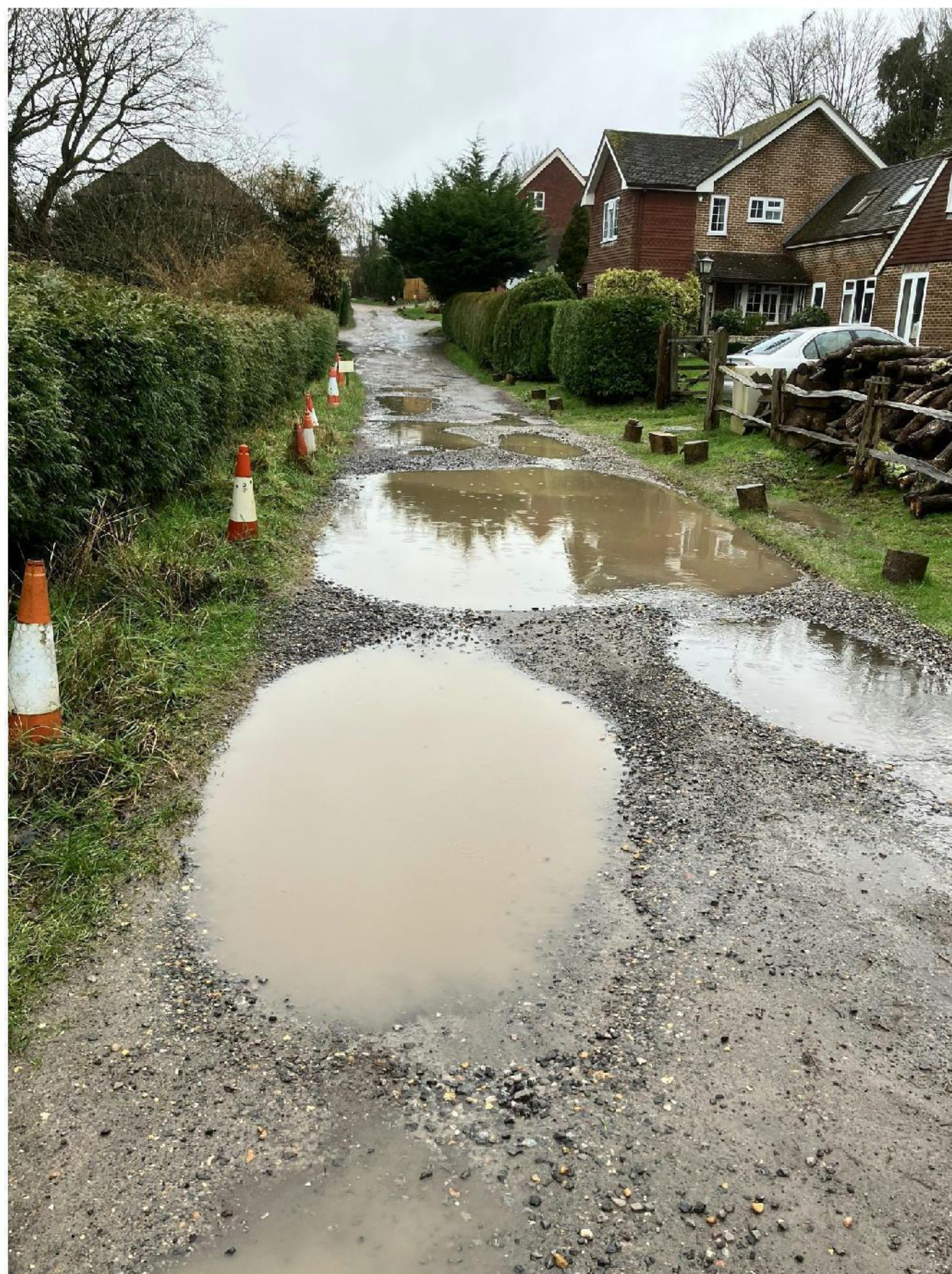
Figure 3: Typical condition of the track (used by pedestrians and vehicles) — extensively flooded, severely potholed, and strewn with loose material. This track does not provide the ‘safe continuous pedestrian access’ described by the applicant.
