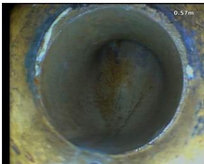
Observation [3]: FRACTURE ON REST BEND
