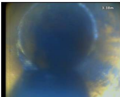
Observation [8]: DROPPED PIPE
