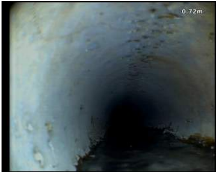
Observation [2]: SCALE BUILD UP
