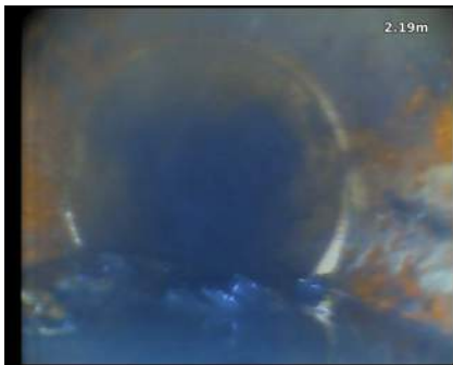
Observation [7]: DROPPED PIPE
