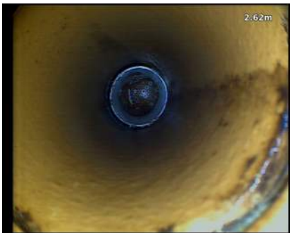
Observation [8]: End Point: WC
