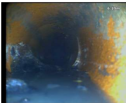
Observation [12]: DROPPED SECTION OF PIPE
