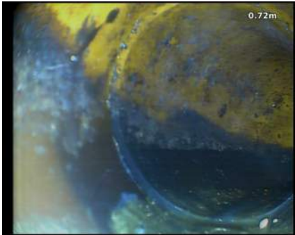
Observation [2]: LINE DEVIATES RIGHT
