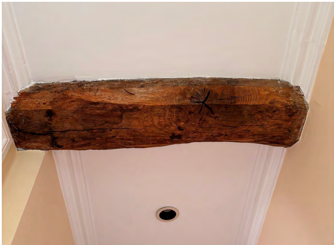
Figure 109: Plate 74 - Beam within the south corridor
