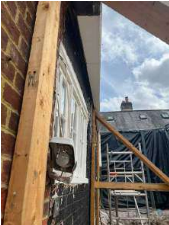
Photograph of the South wall of the original bake house shows sand and cement mortar and partially painted black brickwork not suitable for reuse.
