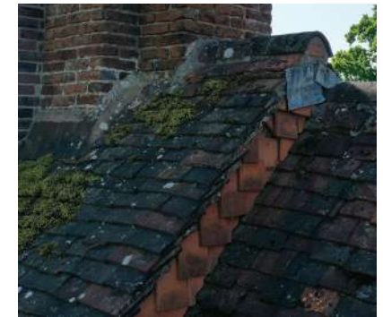
double lap tiles evident at verge
