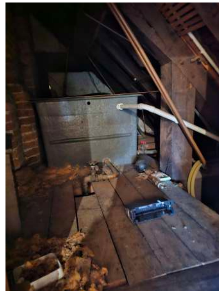
interior of void to south east valley hip of C17th range
