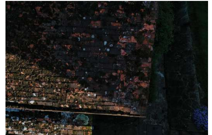
spalling due to moss build up to north lean-to
