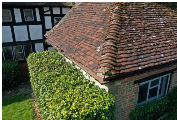
bonnet tiles to hip with mortar lost to bedding
