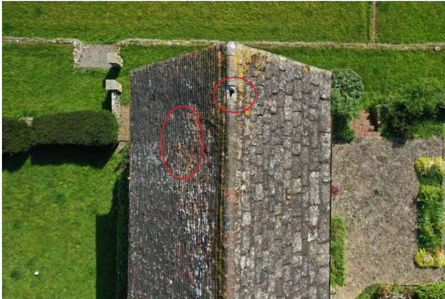
missing tiles and spalling
