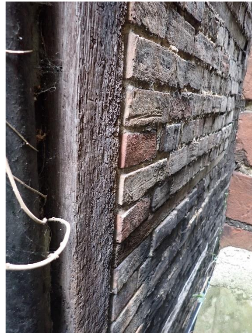
Figure 31: Northern chimney, bricks laid with faces mis-aligned due to proximity of Somners southern chimney, about 200mm
