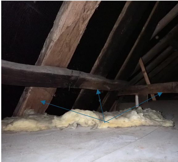
Figure 7: Mixed pattern of smoke blackened and not smoke blackened rafters, collars and eastern side purlin over Bay 1.
