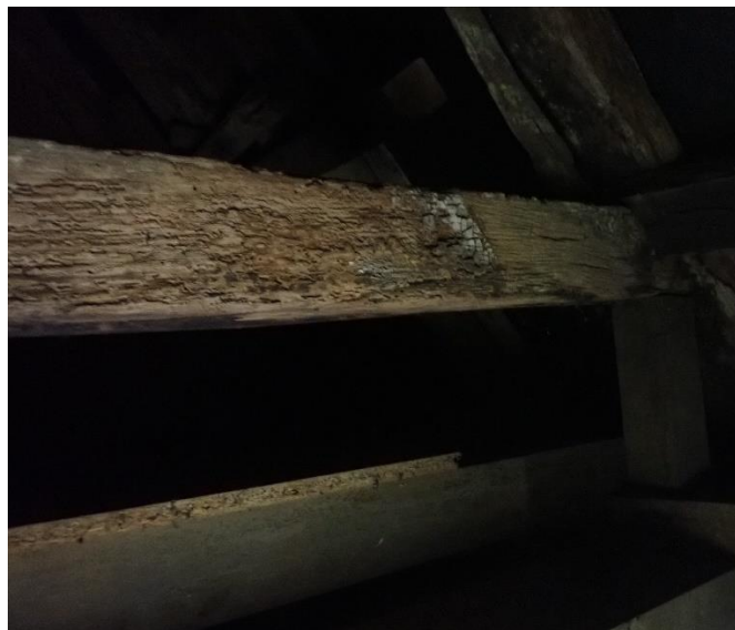
Figure 6: Significant decay pattern on the collar clasping the side purlin, indicating reuse or built against a feature like a masonry chimney stack.
