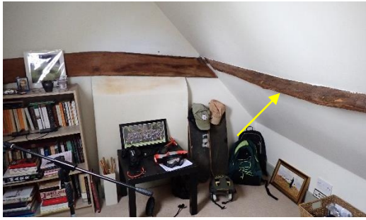
Figure 34: clapsed side-purlin in Bay 6, at loft level.
