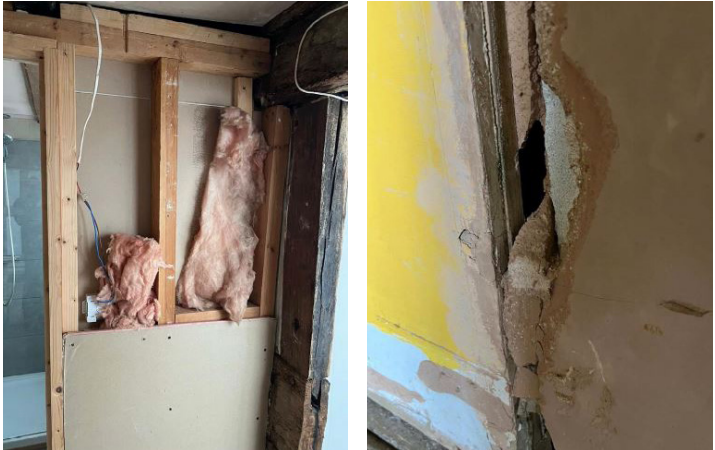
Poor quality bathroom wall build up exposed before demolition Poor quality bathroom wall before demolition
