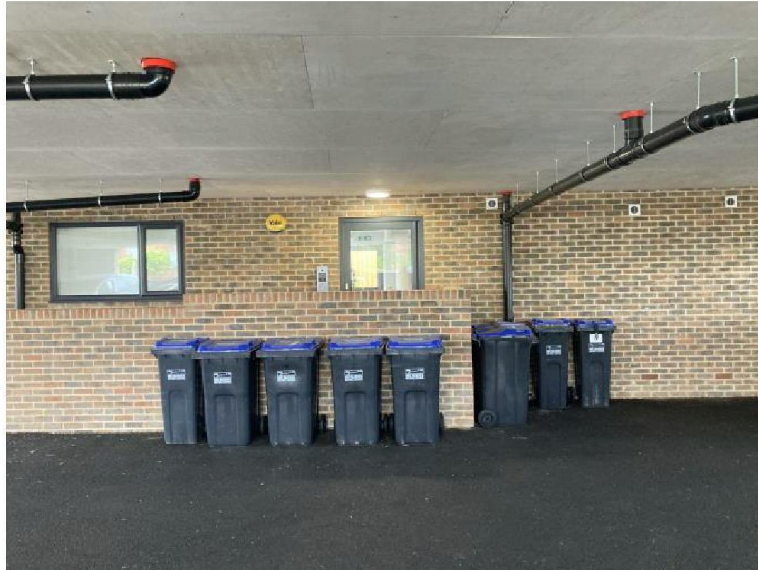
Nine Recycling bins kept within the undercroft
