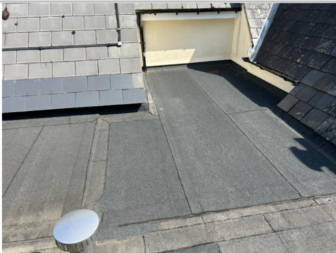
Remedials carried out to area of severe Blisters - 22/06/2026 15:41
