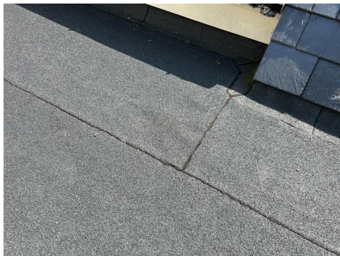
Blister in the area of Remedials - 22/06/2026 15:41
