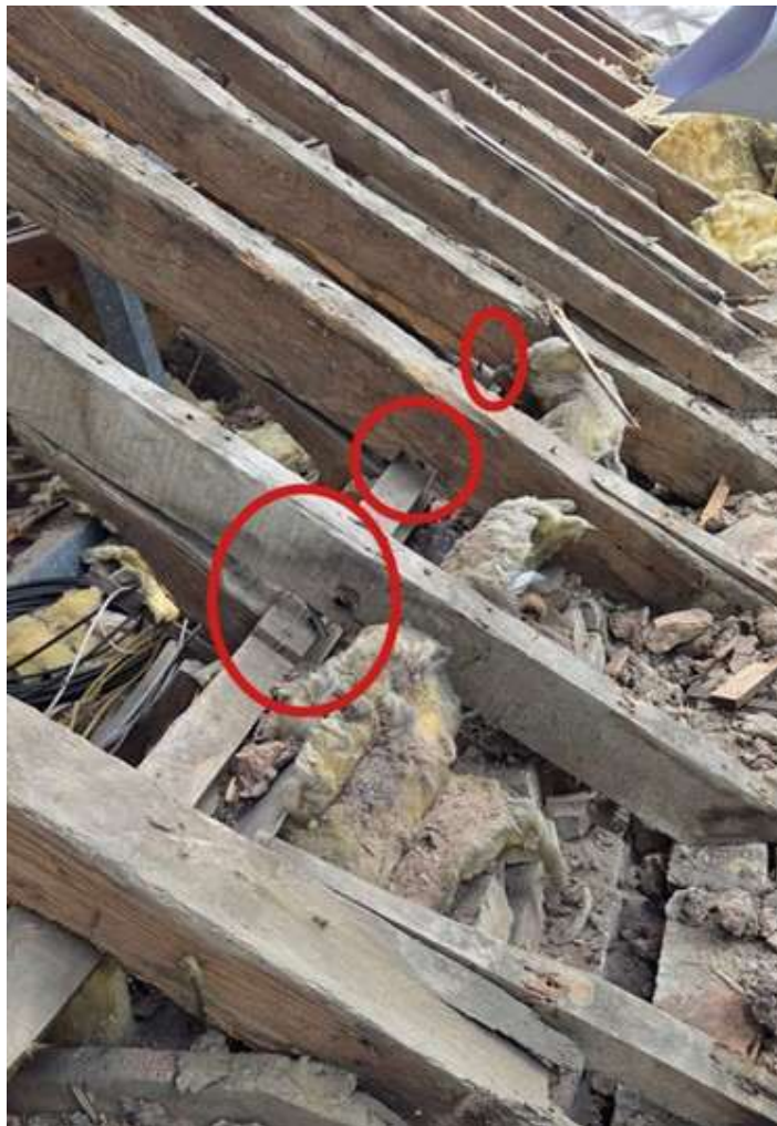
Photograph 21: Gap between rafters and edge purlin
