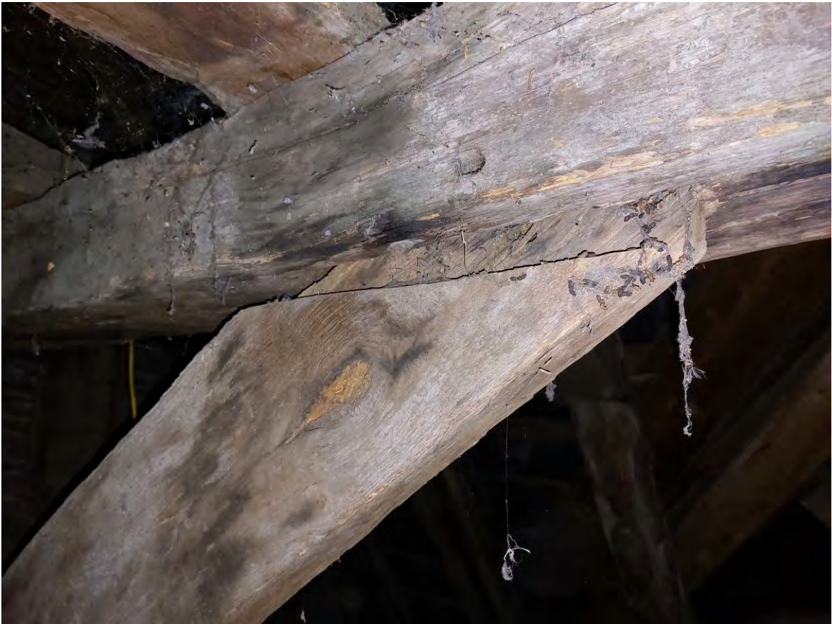
Photograph 7: Dropped brace to be wedged back in place
