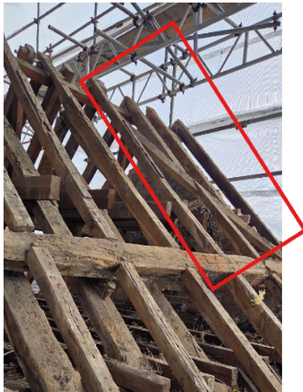
Photograph 20: Discontinued rafters in bay 1
