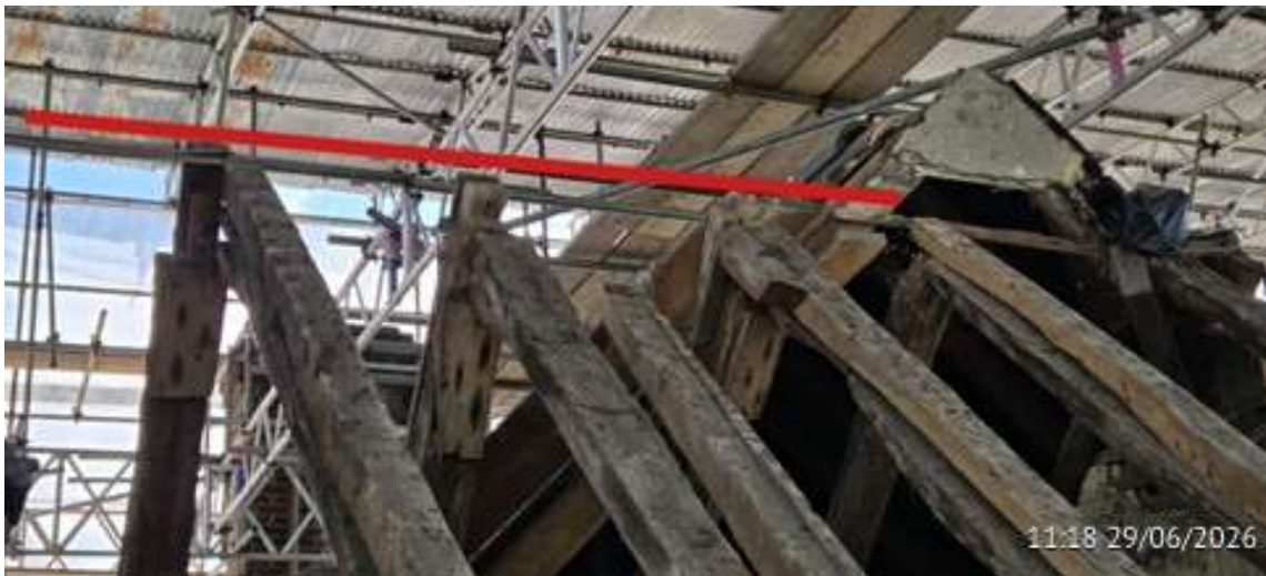
Photograph 17: Ridge beam missing in bay 5
