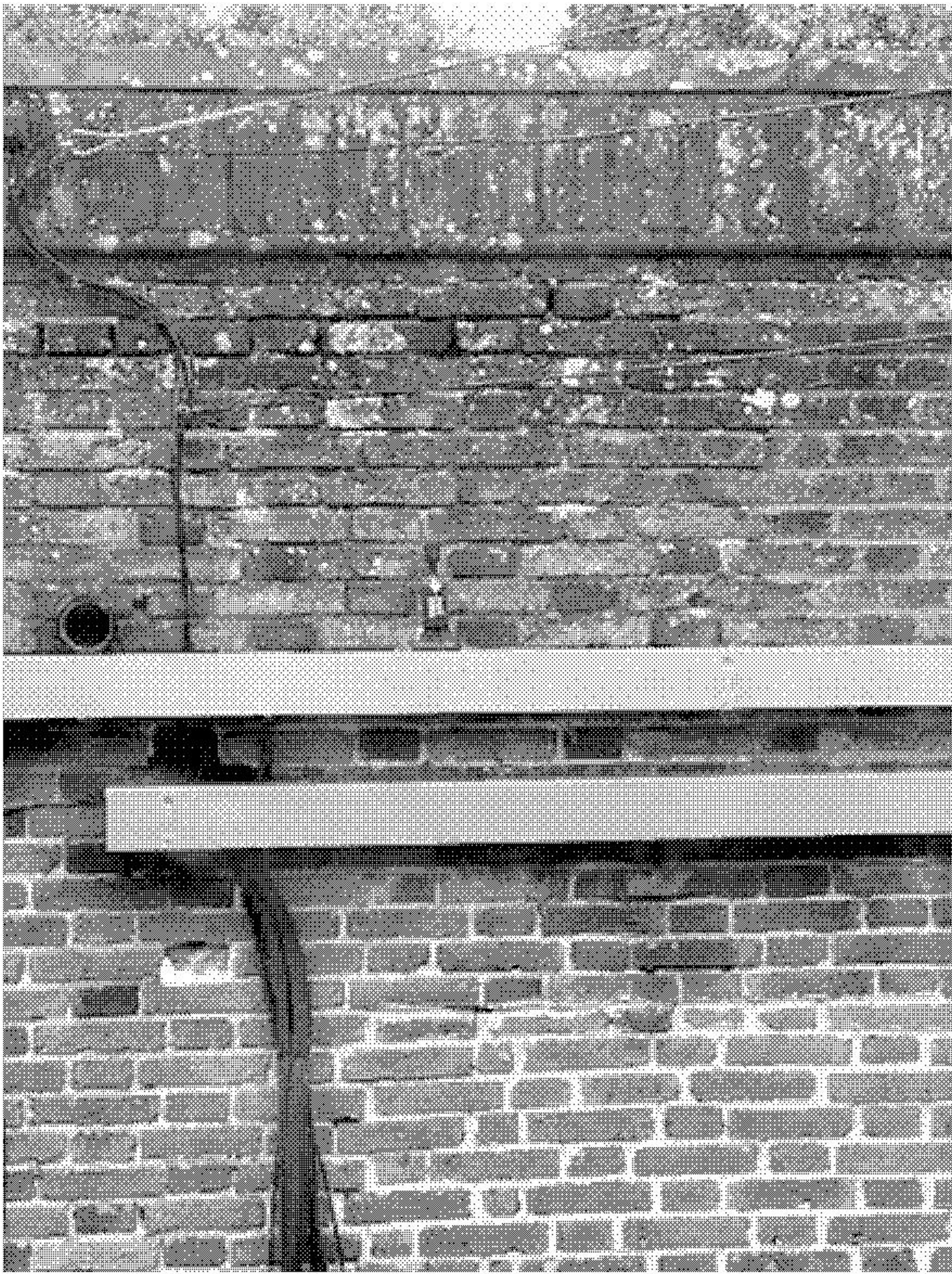
View from side – note large holes and finish
