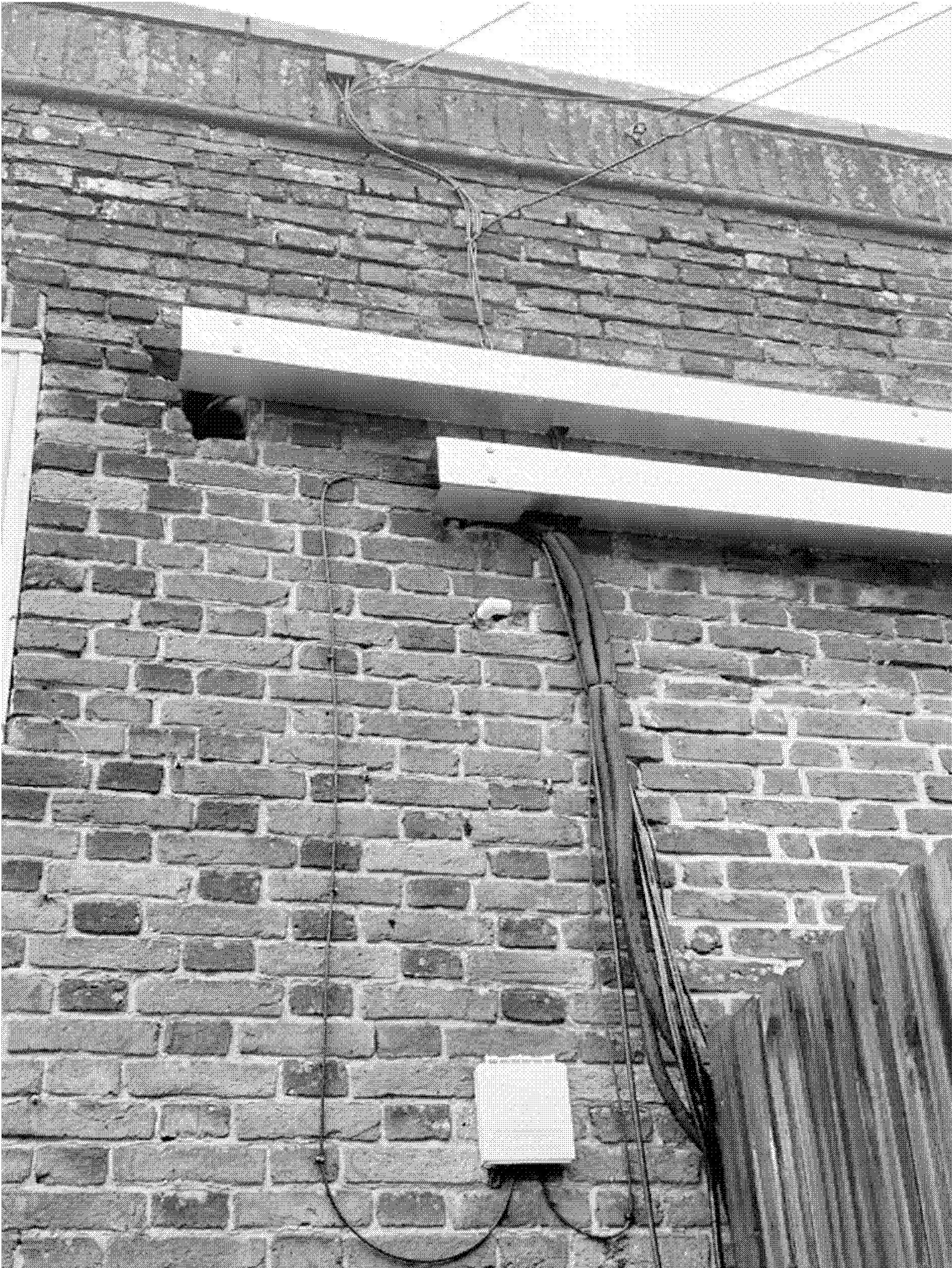
DIY approach of cabling
